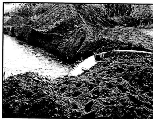
Discharge of water during step-test
