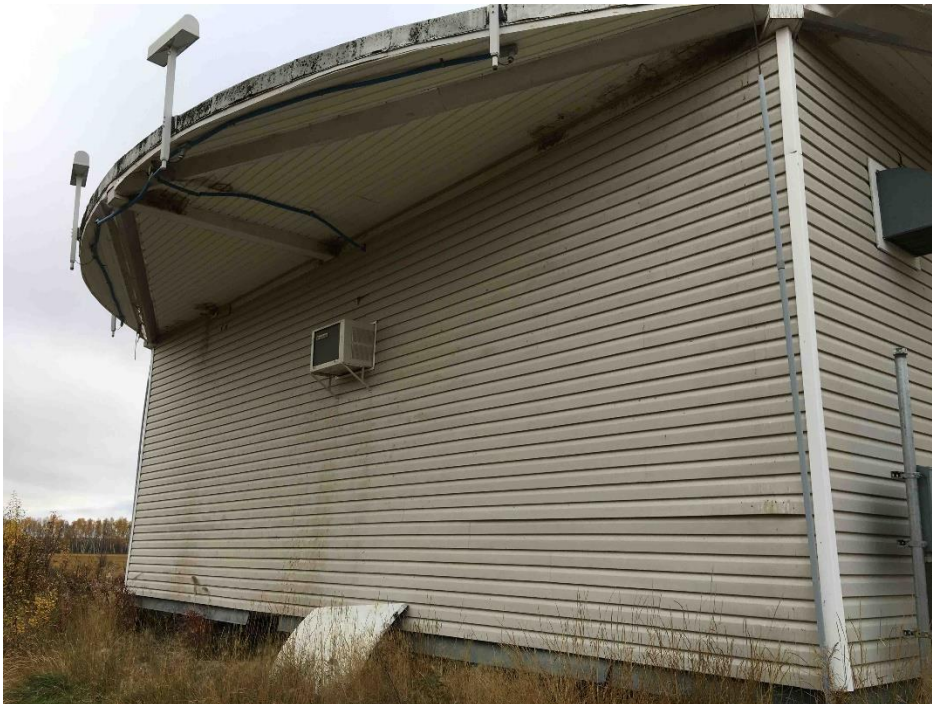
4. GAL VOR building, west façade, showing the window AC unit and vinyl siding.
