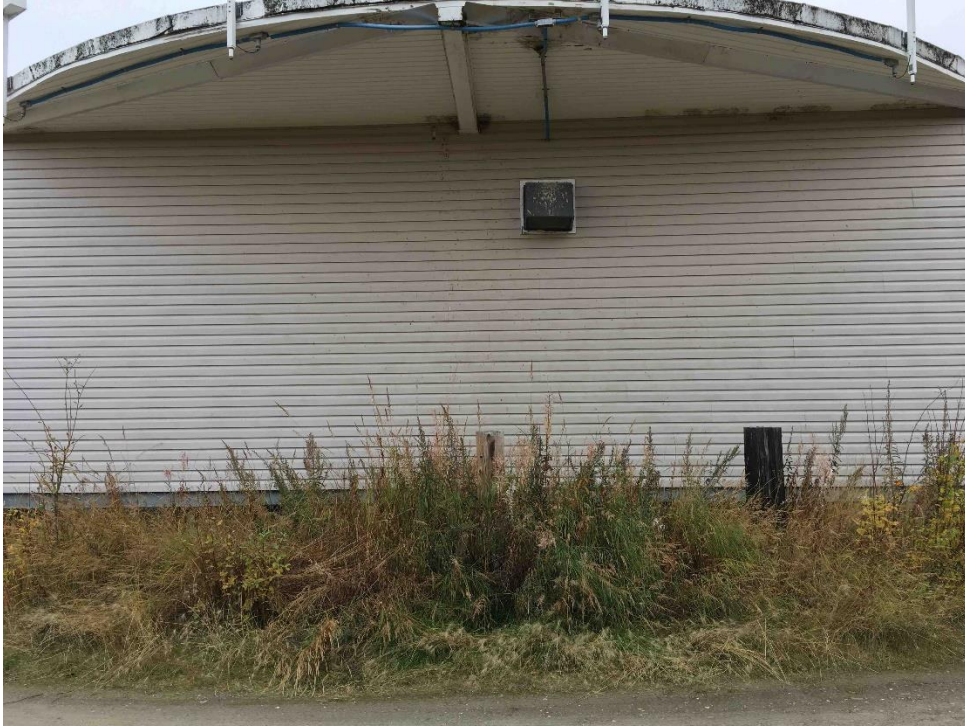
3. GAL VOR building, north (rear) façade, showing vent hood and remnant wood posts from the former air handler.
