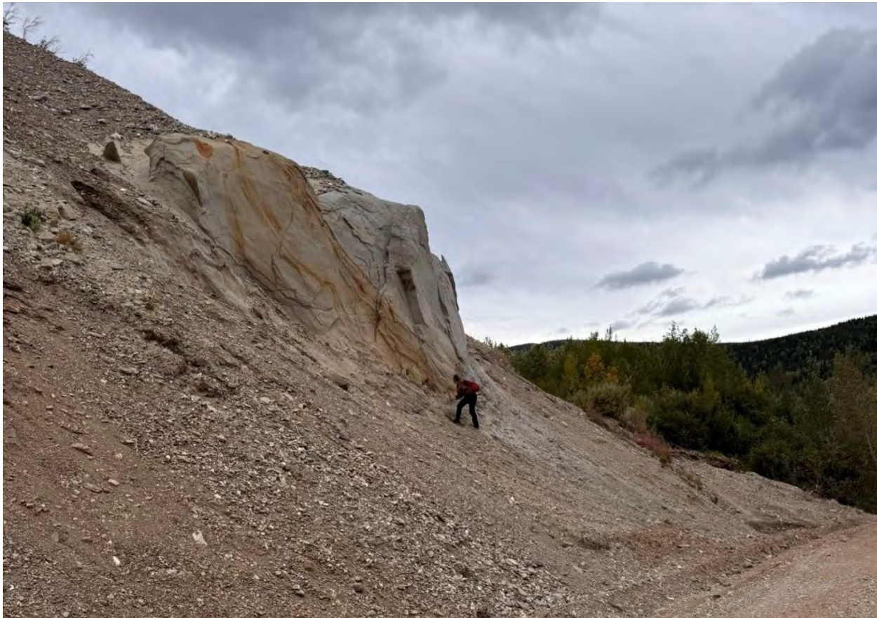
Figure 6: Sandstone in road cut (view north). Note RECON field staff for scale.
