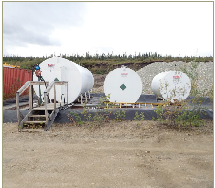
Photo 31. On-site fuel storage with containment, Fortymile Mining District Alaska 2019 (DNR).
