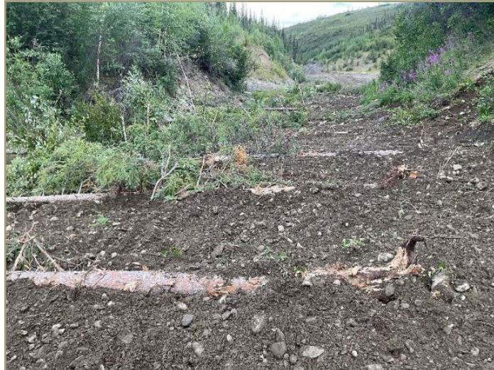
Photo 42. Spruce logs and vegetation transplant mats used to minimize floodplain erosion until vegetation is fully reestablished. From BLM's " Stream Reclamation Basics ."
