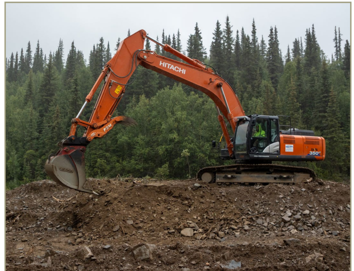
Photo 17. An excavator with a “thumb” is especially useful to pick up and place boulders and logs that are difficult to move with the bucket alone (source unknown).
