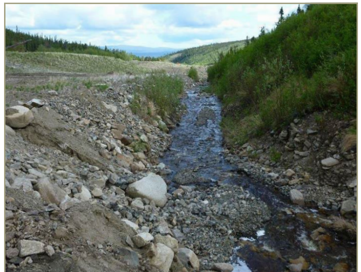
Photo 41. This poorly constructed stream has little to no floodplain connectivity because it likely will not overtop and spread water across its potential floodplain on the left. From BLM's " Stream Reclamation Basics ."
