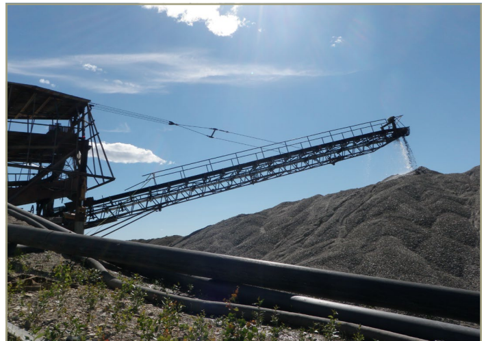
Photo 19. Stacker conveyor, 2013 (DEC).
