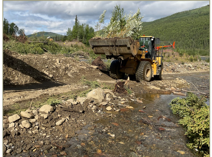
Photo 36. Wheel-loader moving an intact block of soil and vegetation (vegetation mat) from a source (donor) site to an area being reclaimed. This creates “instant” vegetation. From BLM’s “Stream Reclamation Basics.”
