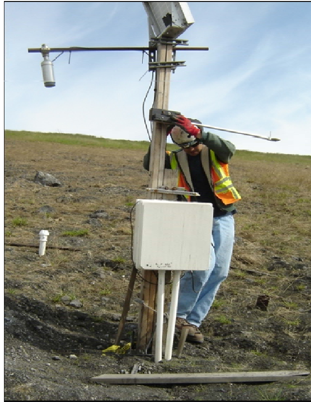
Figure 2.1 West slope station before repairs, person is holding up the net radiometer original location.
