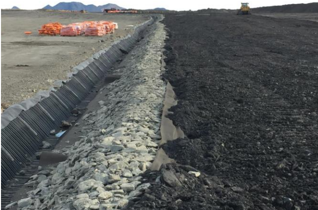
Photo 3 – Looking north, on upper surface of MWD. Drainage channel to the left.
