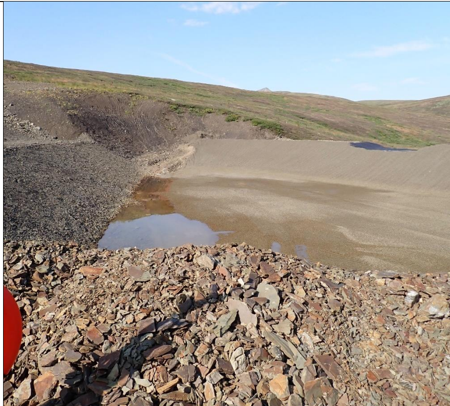
Photo 9: Standing water within the southwestern corner of the Main Dam Seepage Collection area. Standing water has been observed in this location during several inspections.
