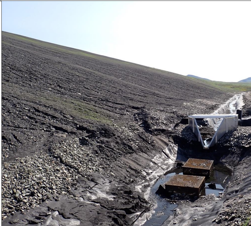
Photo 19: View of ditch that runs adjacent to main WRD. Notice the amount of topsoil that has accumulated within it from erosion.
