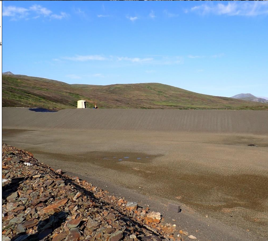
Photo 8: View of the Main Dam Seepage Collection Impoundment looking north. Overall upkeep and maintenance of the facility is exceptional.
