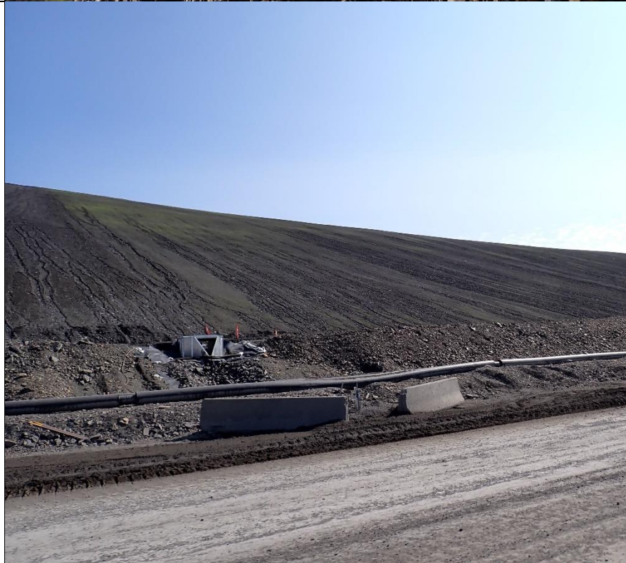
Photo 18: View of rills along main WRD after high precipitation event. Channeling becomes more defined downslope. Recommend using BMPs to re-establish site for seeding.
