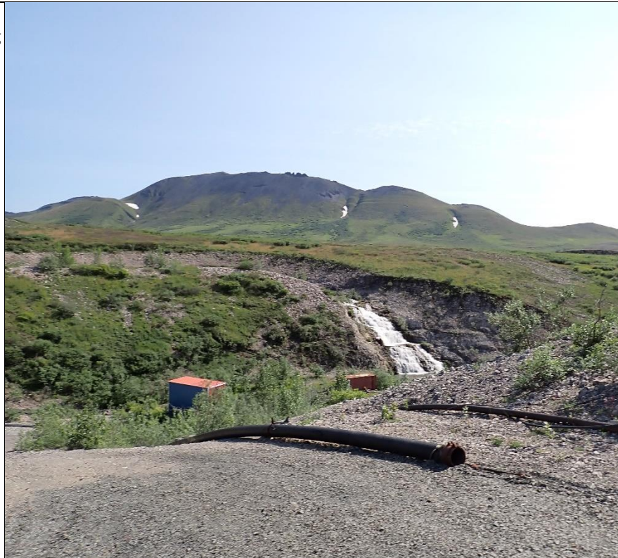
Photo 21: View from atop Bons Reservoir dam looking at the spillway. Below is a pump station for the dam.
