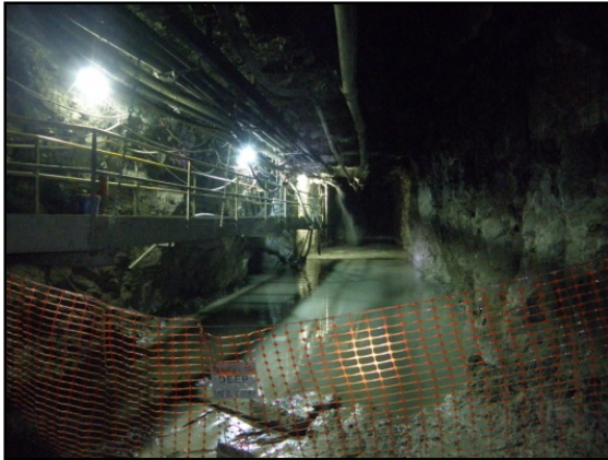
Photo 3: Underground sump for water treatment and reuse.
