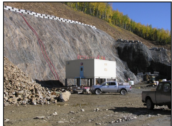
Photo 28: Supporting equipment for the 2150 portal.
