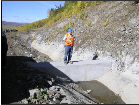
Photo 19: The old north diversion ditch is plugged.
