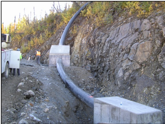
Photo 21: A view of the pipe system for the south new diversion ditch.
