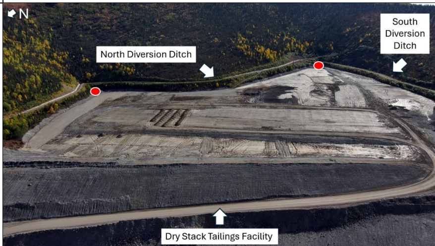
Photo 2: Another view of the DSTF including top and upper shell. Red dots mark areas of Flow Through Drains.
