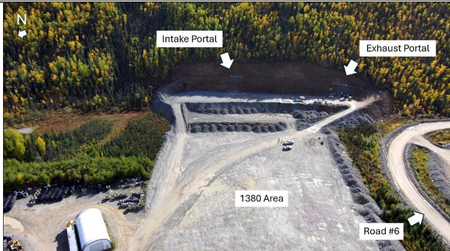
Photo 8: View of 1380 Area progress including locations of Intake and Exhaust portals. Boneyard to the left.
