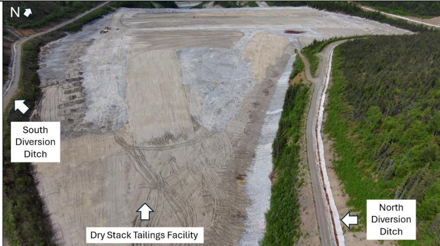
Photo 1: Dry Stack Tailings Facility (DSTF). View from the upper DSTF looking at the expansion extents.
