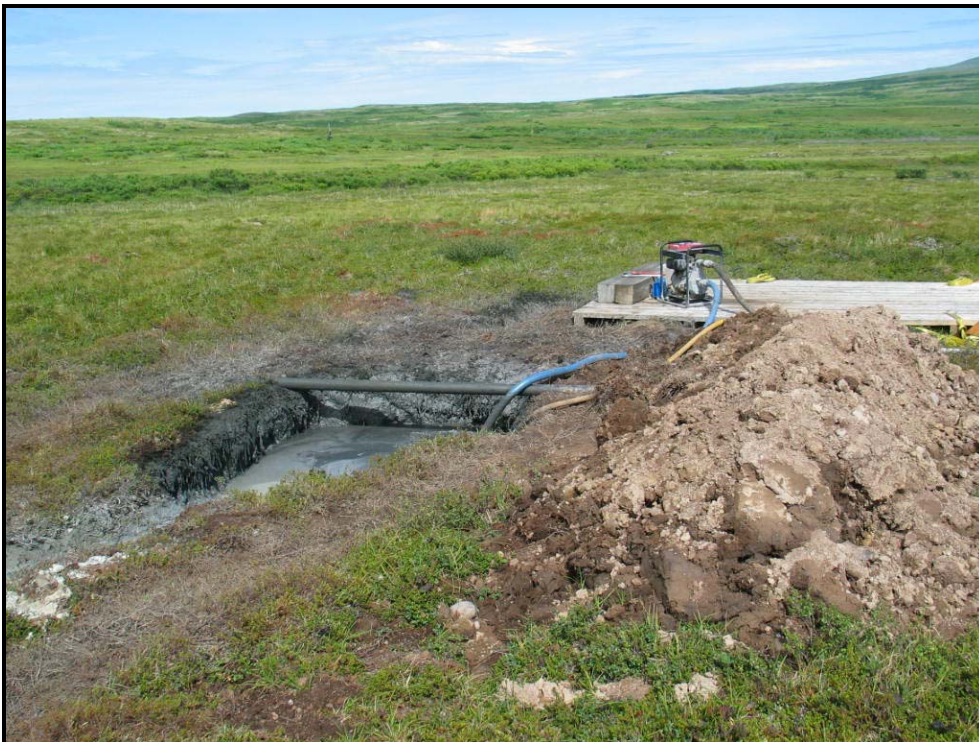
Photo #19. Sump at drill #6.
