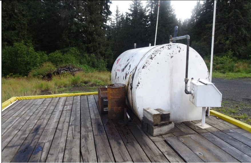
Photo 12: Fuel Tank at Laydown Yard near Helicopter Landing Zone. Note the duck pond liner.
