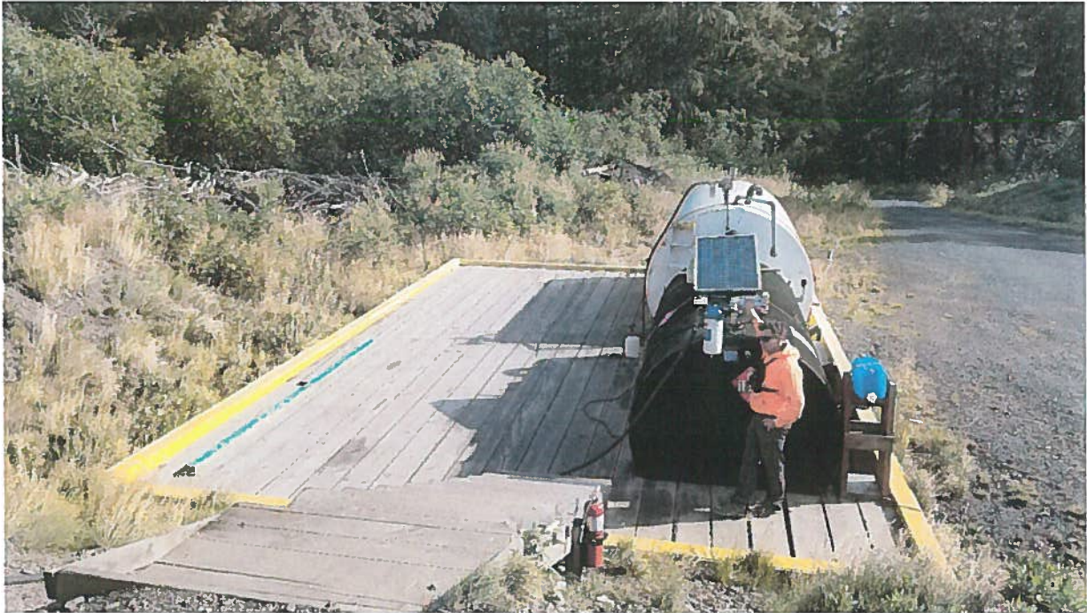
Photo 1. Fuel Station at the Glacier Creek Laydown. Tanks were emptied and winterized in October 2019, unused in 2020.
