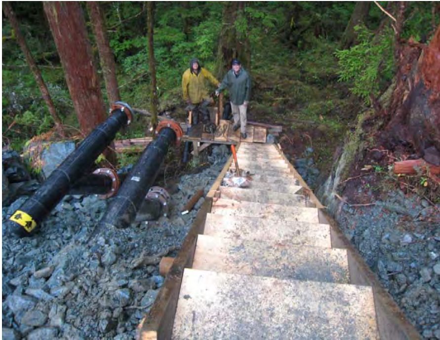
Photo 13. HDPE pipes exiting water treatment facility/sediment ponds and leading to Land Application Area.
