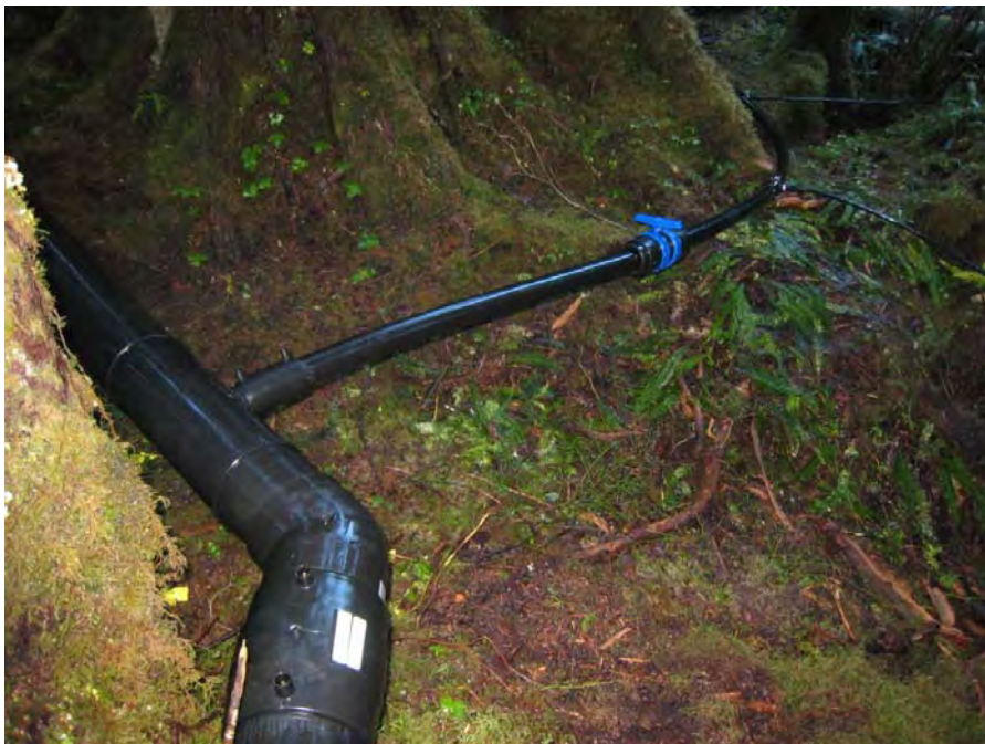
Photo 14. Land Application Area, distribution system with 6-in. main line connecting to 2-in. pipe that services drip emitter lines for a single land application zone.
