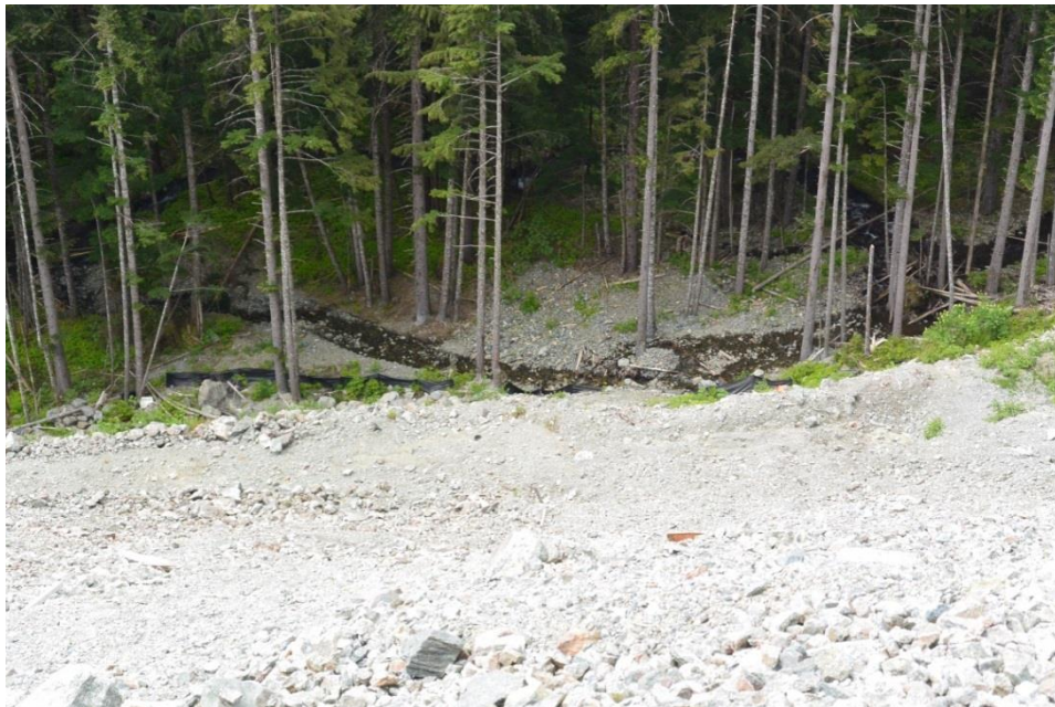
Figure 7 The silt fence running between the Comet Wasterock Pile and Ophir Creek was partially buried.
