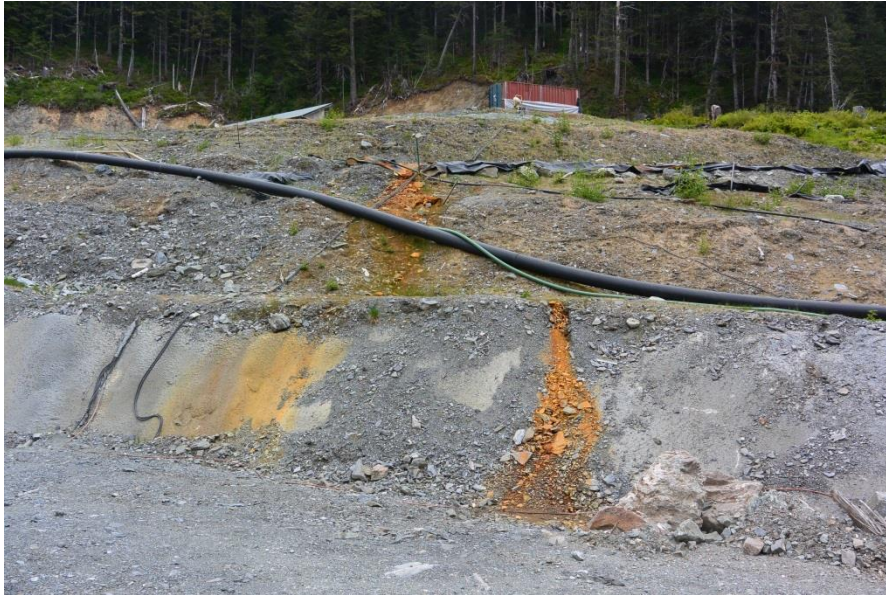
Figure 3 Orange staining below the Tailings Treatment Facility Dam.
