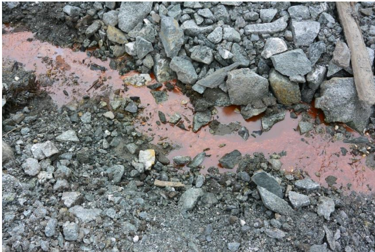
Figure 5 The discoloration in this seep appeared to be the result of organic decomposition and digestion by iron bacteria.
