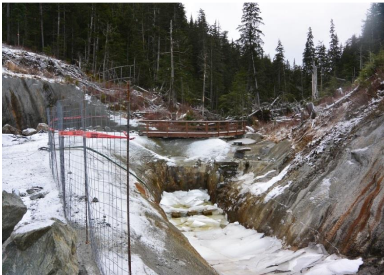
Figure 3 Plunge pool. Note the new guarding.
