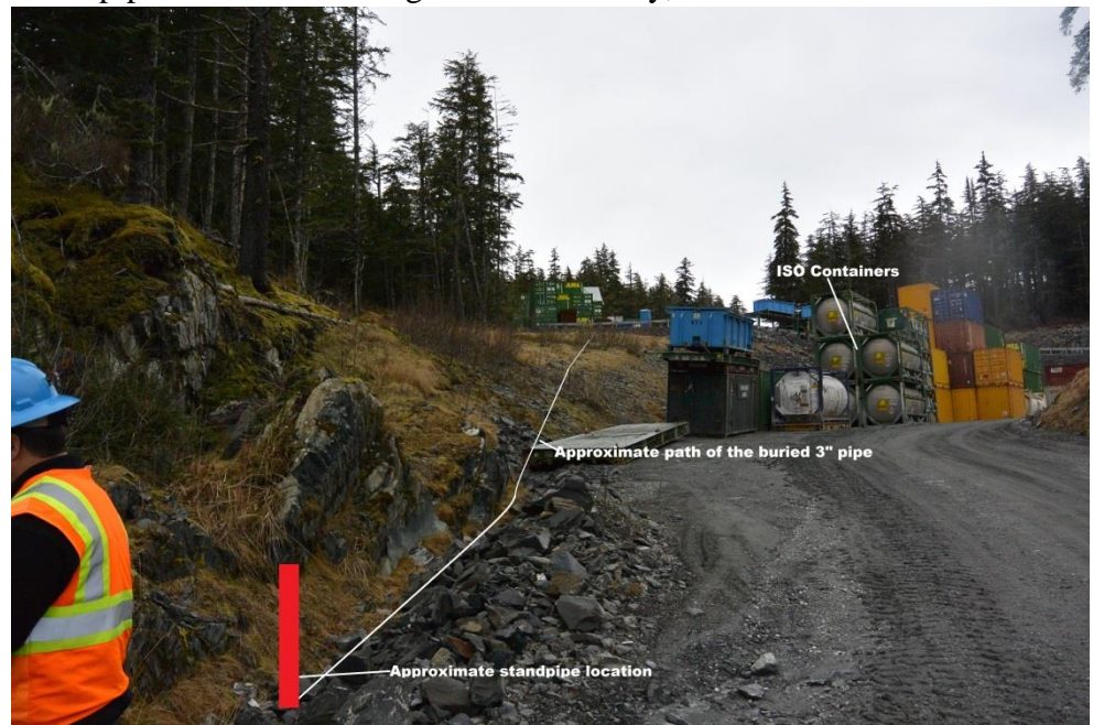
Figure 11 The approximate path the buried 3" pipe will take to the proposed tank farm. Note the ISO containers next to the road.
