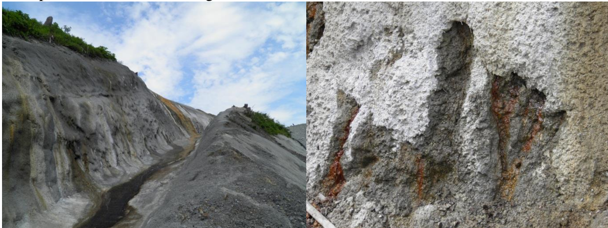
Figure 10 Spillway and shotcrete covering the GP. Low pH water seeping through the shotcrete is eroding it.
