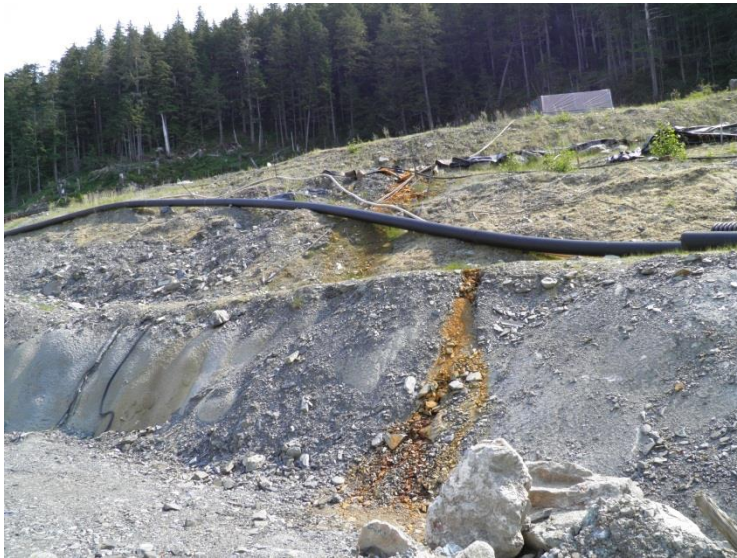
Figure 11 Staining beginning to show near the east end of the dam.
