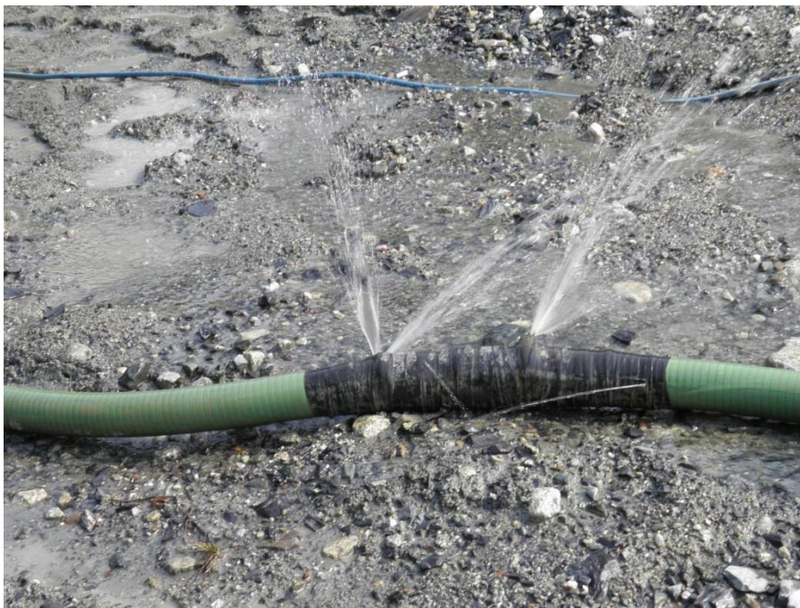
Figure 4 The hose had been mended, but the repair was insufficient.
