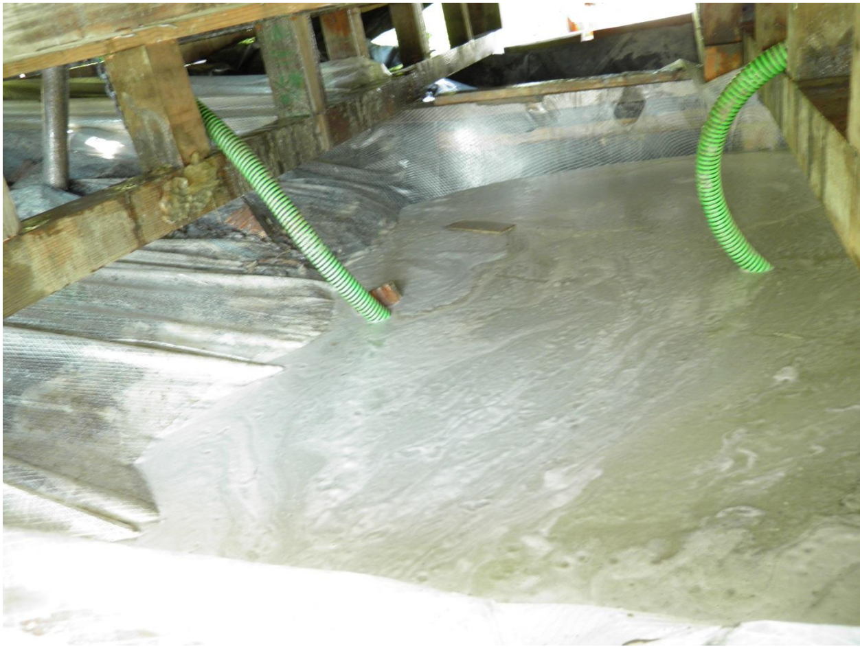
Figure 15 The thin layer of plastic separated the drill water and the ditch directly below.
