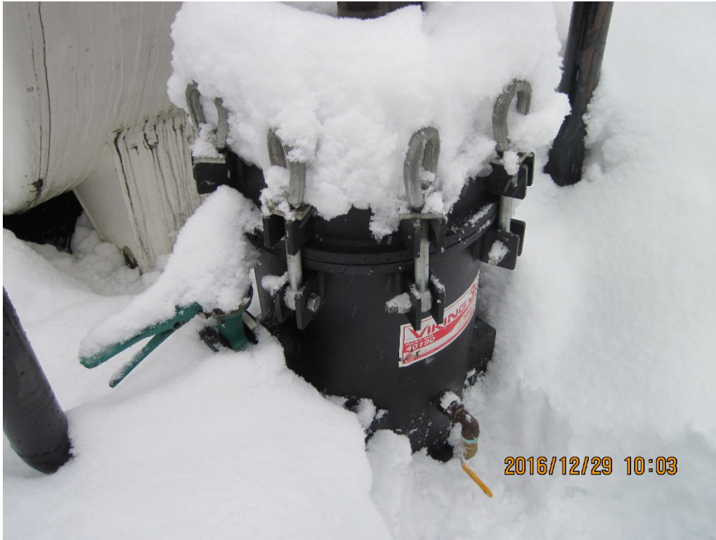
Photo 2. During refueling, diesel from the isotainer flows through this filter, located on the back of the day tank.
