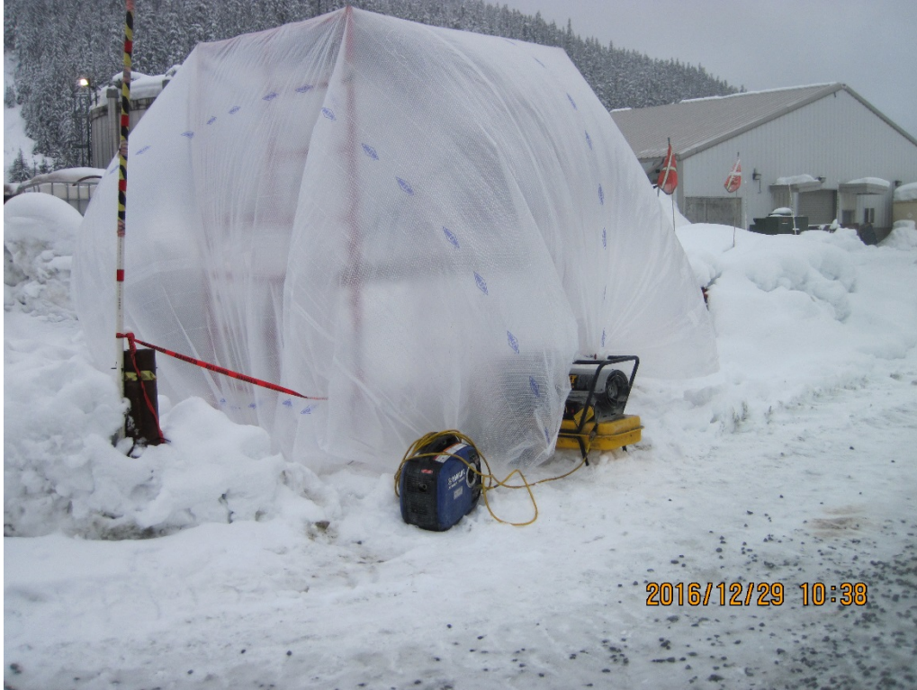
Photo 6. Defrosting the OWS. Crews assembled a tent around the OWS to speed up the defrosting process. During the spill, the OWS was frozen and multiple feet of snow covered the ground.
