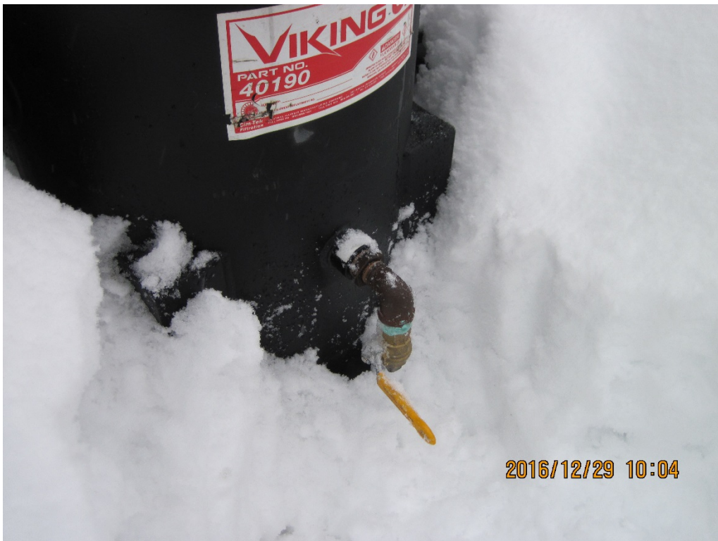
Photo 3. Ball valve on the filter was in the “open” position, allowing diesel to escape from the filter during refueling. The valve has since been plugged and the orientation of its handle has been changed to prevent falling snow/ice from opening it.
