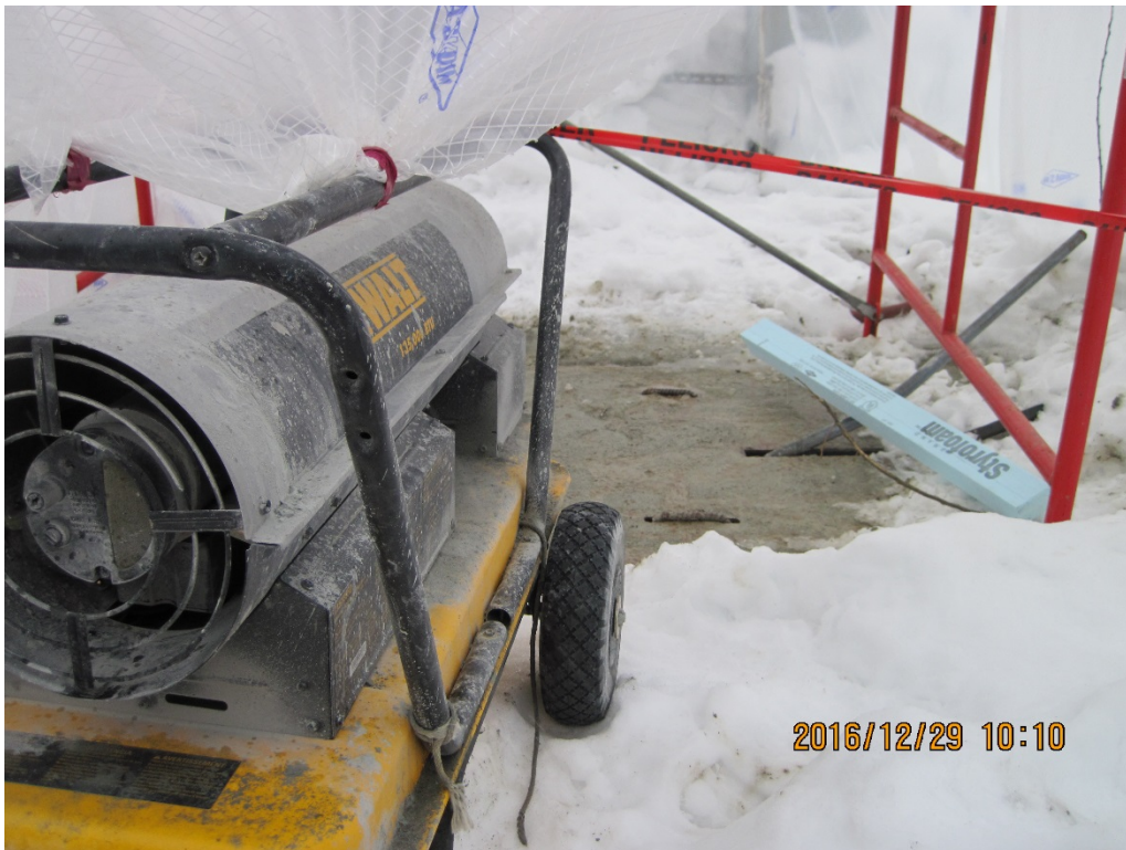
Photo 5. Defrosting the oil/water separator (OWS). The OWS is a metal tank in a concrete container located beneath the recently exposed cover on the ground. Ice filled the OWS, rendering it inoperable.
