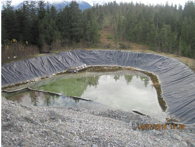
Photo 16. An existing settling pond at Pit 4 will collect stormwater runoff from the waste rock pile.
