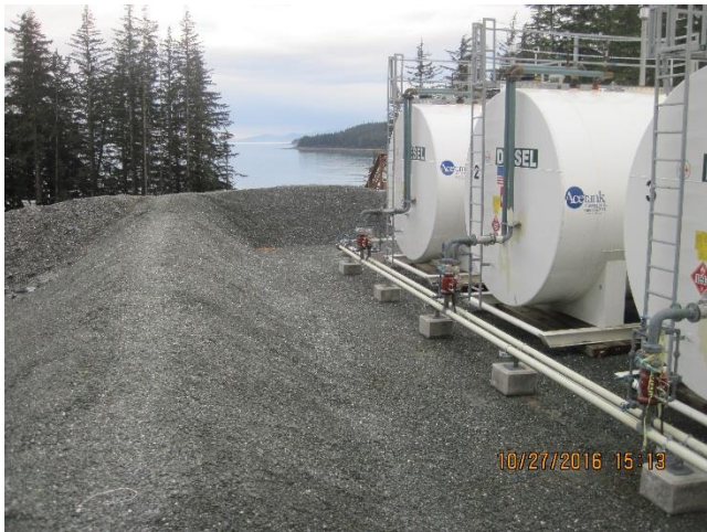
Photo 23. Seven 50,000-gallon double walled fuel tanks.
