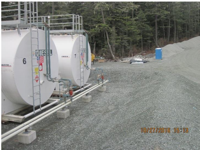
Photo 24. Fuel tanks are placed on a HDPE lined and bermed gravel bed.
