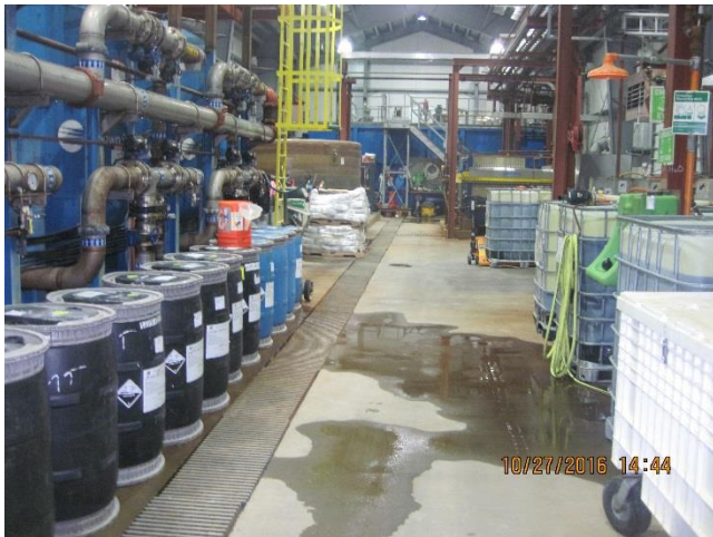
Photo 20. The TTF water treatment plant
