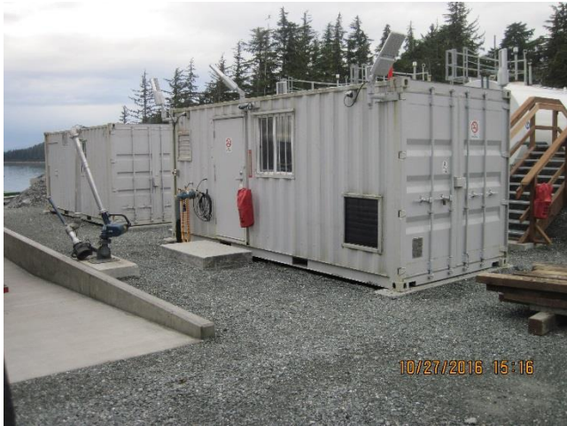
Photo 25. The fuel depot pumping station will transfer fuel from the tanks to a fuel truck.
