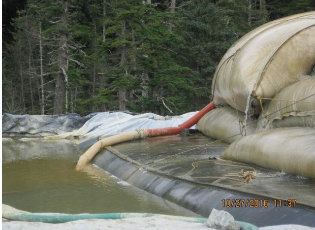
Photo 4. Sediment dewatering bags at the Comet water treatment plant.
