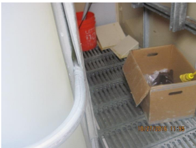
Photo 6. A storage container with secondary containment.
