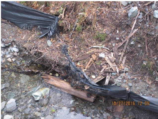
Photo 12. Upper Sherman Creek Bridge silt fencing is torn.
