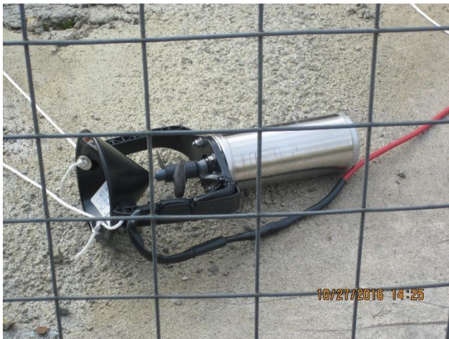
Photo 18. A water agitator at the TTF dam plunge pool.
