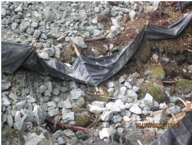
Photo 11. Upper Sherman Creek Bridge silt fencing pushed over.
