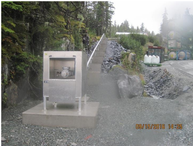
Photo 29. Fuel transfer pipeline from the Kensington port to the fuel depot.
