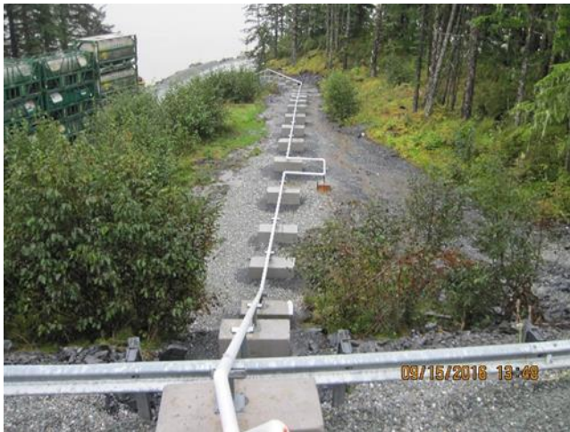
Photo 23. The fuel transfer pipeline installed from the Kensington port to the fuel depot.
