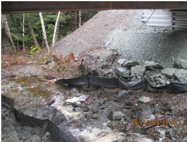
Photo 11. Riprap and silt fencing installed along both bridge abutments (Lower Sherman Creek).
