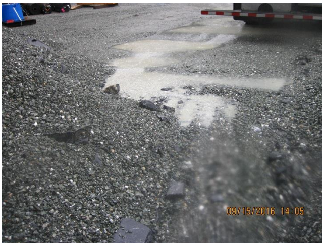
Photo 27. Stormwater ponding and flow paths formed in the gravel parking area of the fuel depot.
