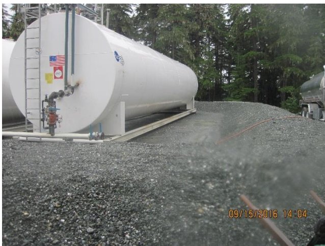
Photo 24. Crushed X-ray reject rock used to construct the berms and gravel layer.
