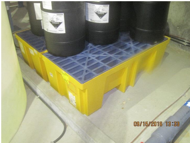
Photo 20. TTF seep plant's secondary containment for chemicals.
