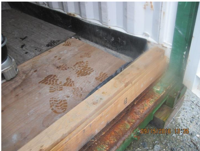
Photo 21. TTF water treatment plant storage container with secondary containment.
