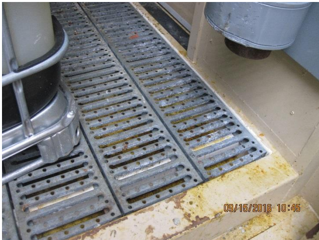
Photo 5. Comet water treatment plant storage container.
