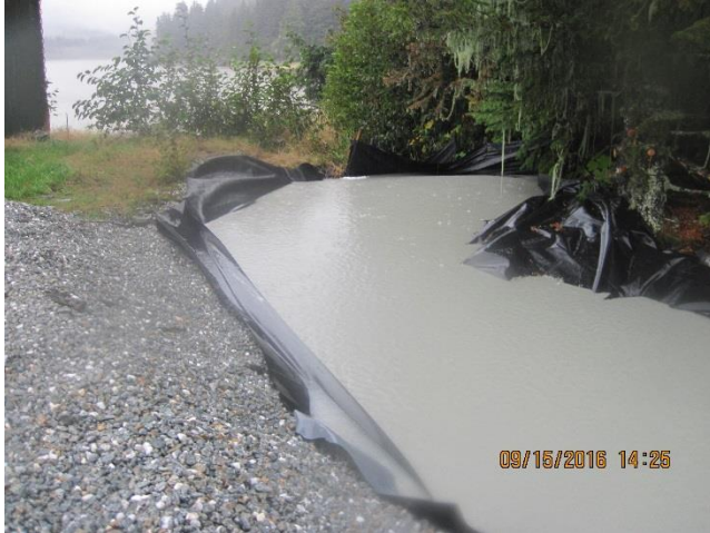
Photo 31. The sump and silt fencing should be frequently monitored at the Kensington port.
