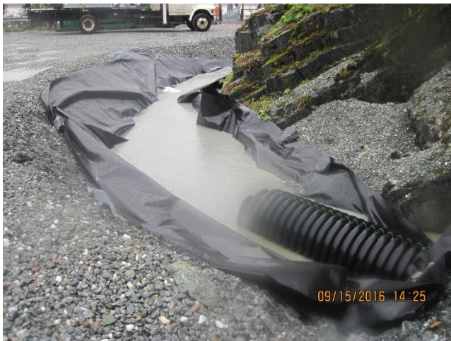
Photo 30. Kensington port lined sump collecting stormwater runoff.
