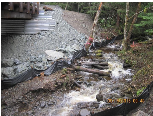
Photo 12. Silt fencing installed to capture stormwater runoff entering upstream of Lower Sherman Creek.
