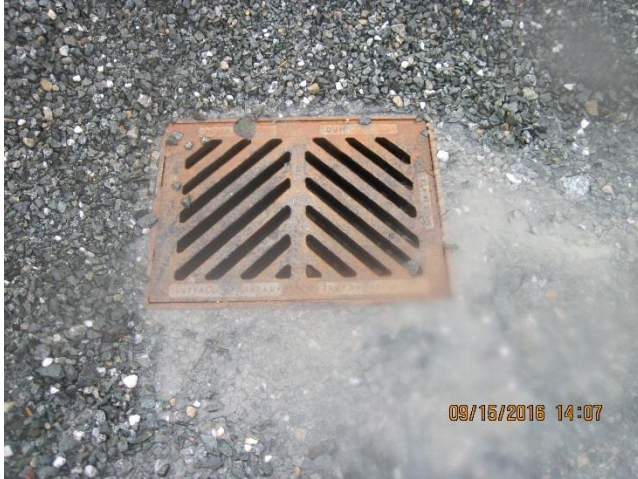
Photo 25. Stormwater drain in fuel depot.
