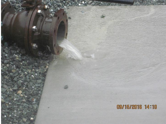
Photo 28. Stormwater drain needs extend out past the fuel depot's concrete walkway.
