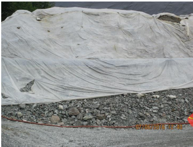
Photo 24. Pit 4 GP liner tears and a section of the liner partially uncovered.
