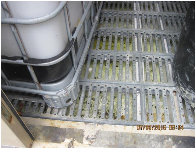
Photo 11. Storage container with secondary containment.
