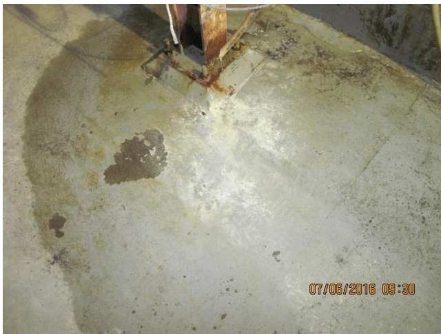
Photo 6. White material buildup observed on the sealed nonporous concrete floor.
