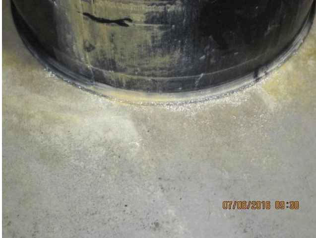
Photo 7. White material on the concrete floor of the Comet water treatment.
