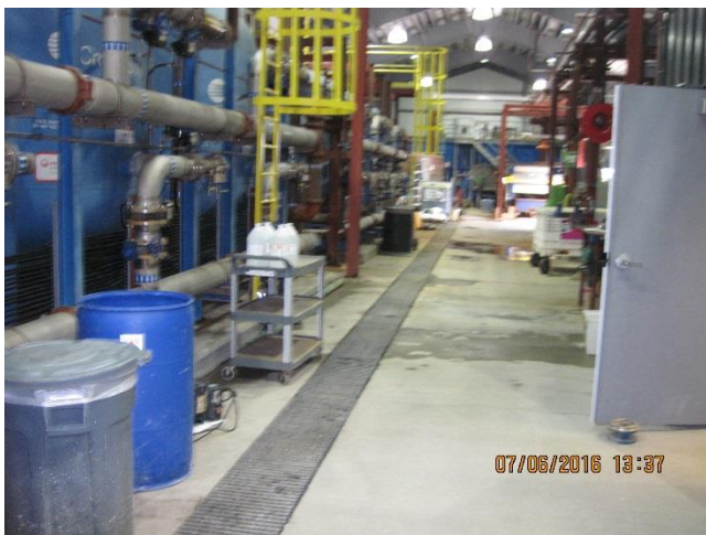
Photo 30. TTF water treatment plant.
