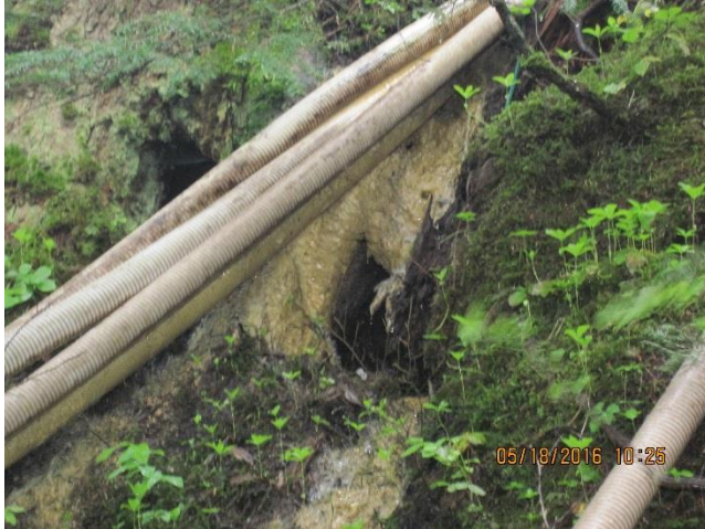
Photo 10. White material was present below the leaking outfall hose.
