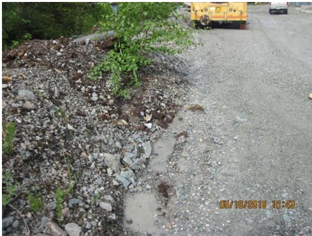
Photo 8. Image of the washed out diversion ditch behind the Comet Water Treatment Plant.
