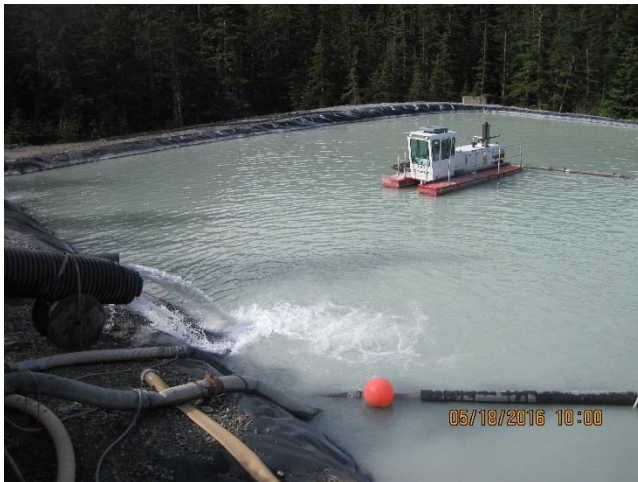
Photo 5. Suction dredging process underway at Pond-1 of the Comet Water Treatment Plant.
