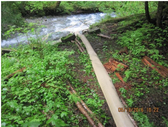
Photo 11. Collapsible water line at the Sherman Creek outfall.
