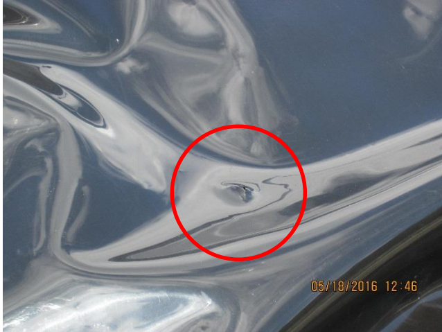
Photo 19. Puncture in a liner used for covering GP material at the Mud Dump.
