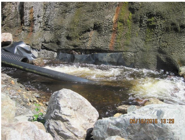
Photo 24. Upper Slate lake bypass and TTF water treatment plant plunge pool.
