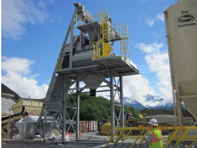
Photo 16. Pug Plant at Pit 4 is not online.
