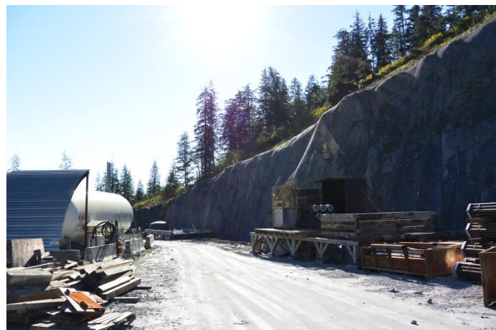
Figure 7 High wall and propane tank.
