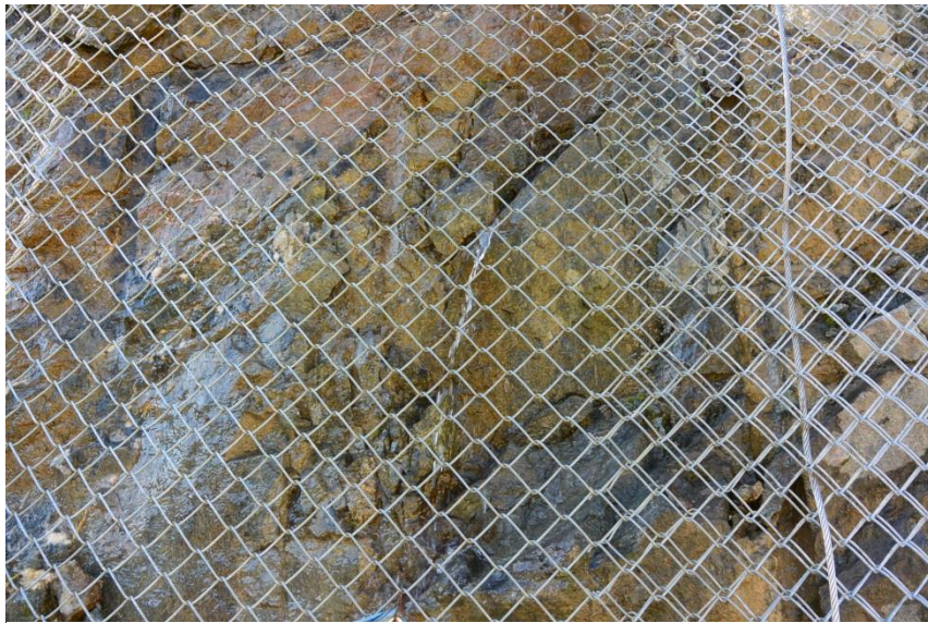
Figure 8 Water seeping from a crack in the high wall.
