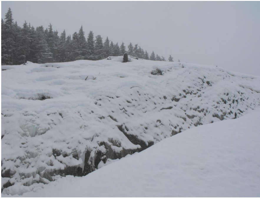
Figure 5 Large ice formations have grown (left side of picture) due to ground water seeping and freezing near the shotcrete. Looking northwest.
