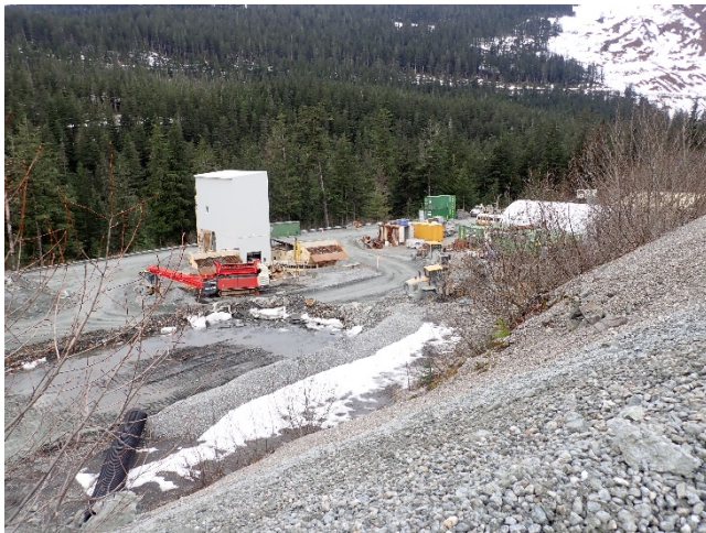
Photo 5. The pug plant.
