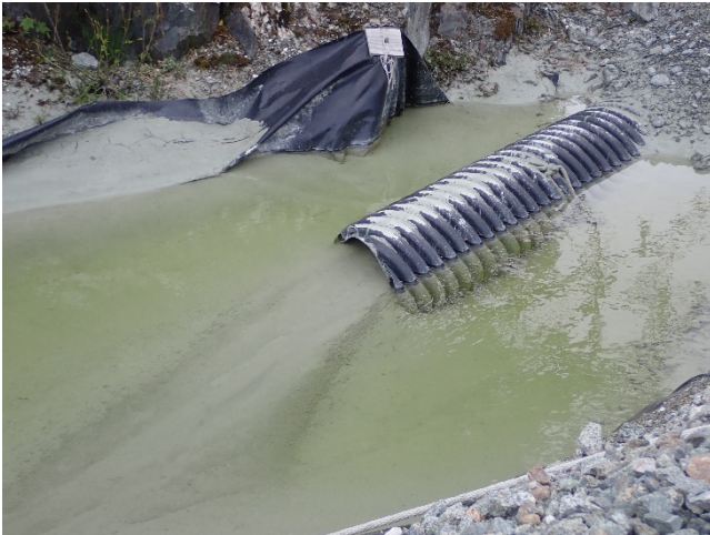
Photo 20. Nearly blocked culvert at port facility settling ponds.
