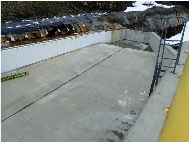
Photo 24. ARD seepage into spillway.
