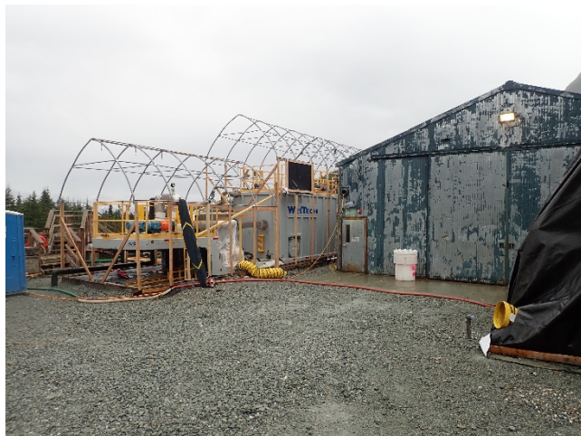
Photo 9. Mobile wastewater treatment plant.
