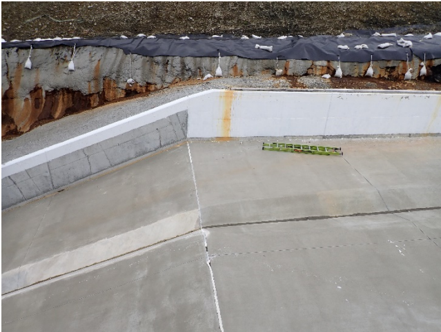
Photo 23. ARD seepage into spillway.
