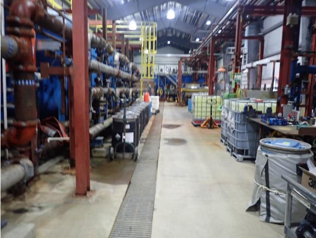
Photo 18. The TTF water treatment plant.
