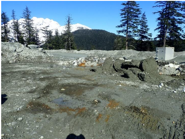
Photo 16. Additional waste rock for the stage 3 dam construction activities will be staged at Pit 7.
