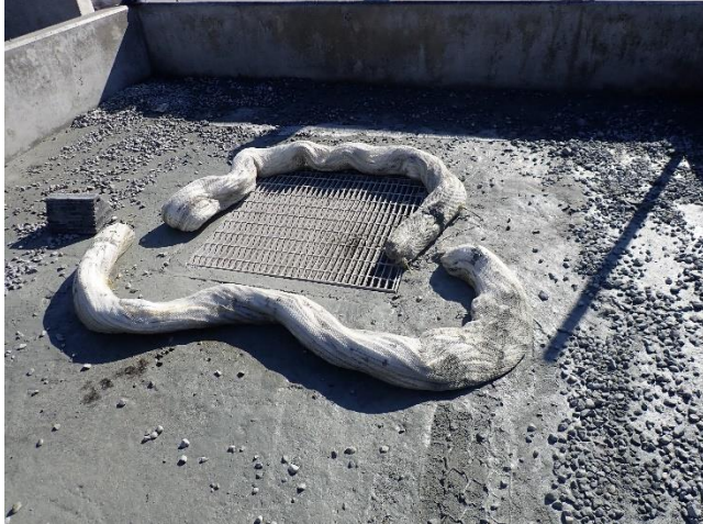
Photo 25. A hydrocarbon contamination boom was placed around the fuel depot's refueling pad's drain to capture small fuel spills.
