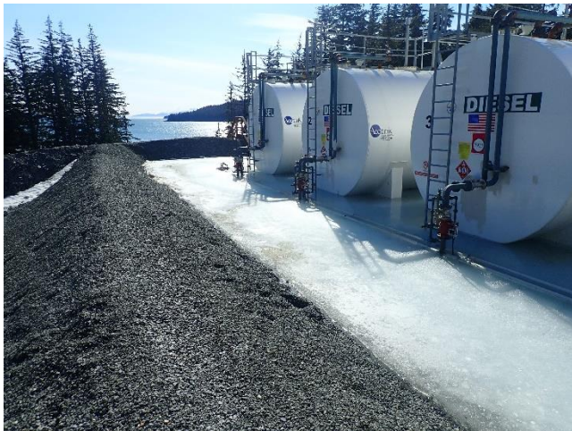
Photo 22. The fuel depot.
