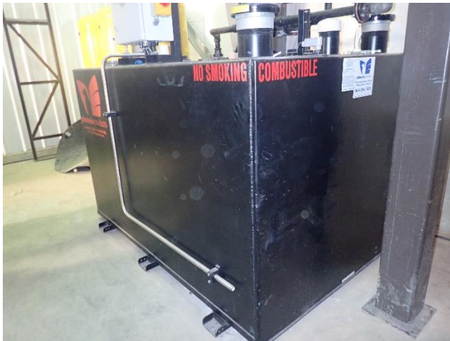
Photo 13. 1,000-gallon fuel tanks are now staged behind all four new generators.
