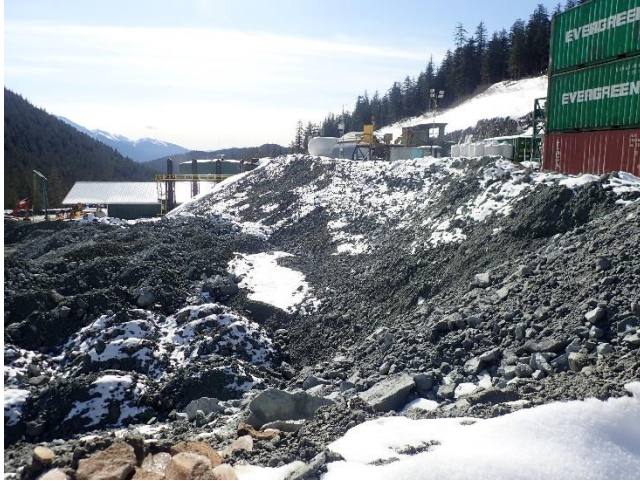
Photo 12. Coeur continues to remove waste rock from the Kensington development pile for the TTF dam expansion.
