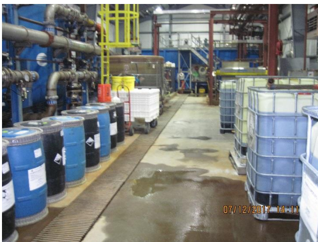
Photo 15. TTF water treatment plant.
