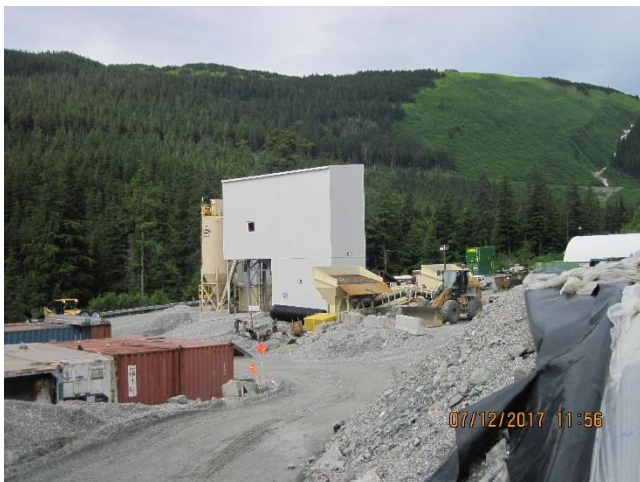
Photo 12. Pug plant at Pit 4.
