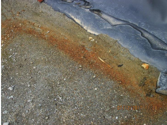
Photo 10. The reddish-stained ground may be a result of ARD water spillage.
