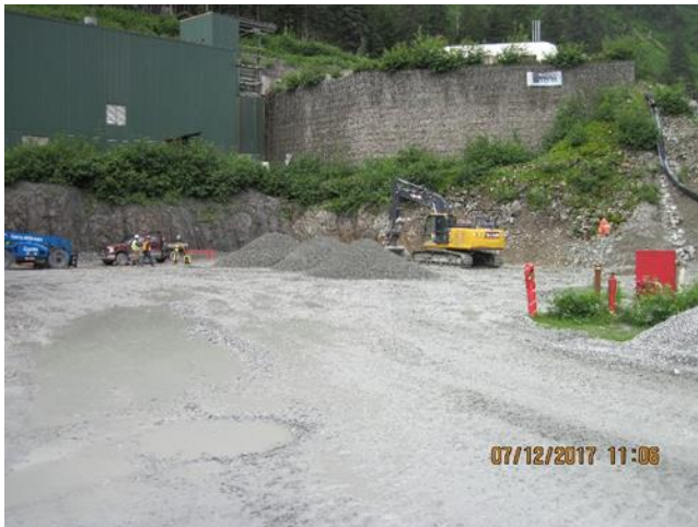
Photo 9. Contractors have begun construction of the foundation pad for the four generators at the mill.
