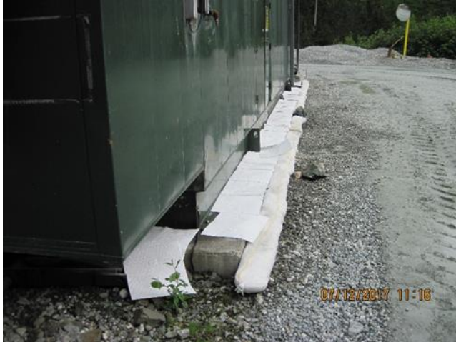
Photo 7. Generator 7 is where 5 gallons of diesel fuel leaked out onto the ground (Image 1 of 2).
