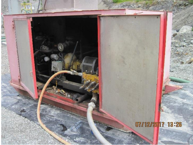
Photo 16. A generator for a geotechnical drilling pad is staged in the southern TTF area.
