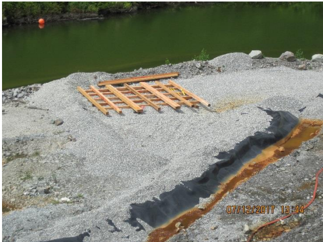
Photo 18. Staged lumber for a geotechnical drilling pad in the northern TTF area.
