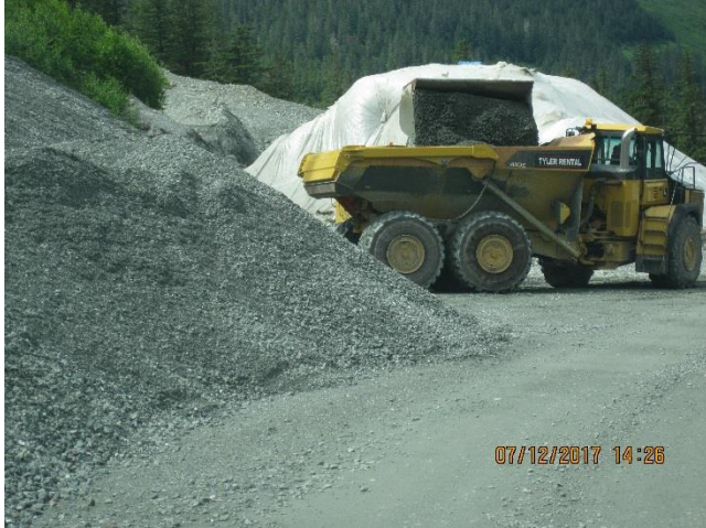
Photo 19. Gravel from Pit 7 is being utilized as a subbase for construction at the Mill.
