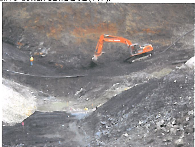
PHOTO 4: VIEW OF TRENCH FROM FLUME. NOTE LOW SPOT ON WEST SIDE OF TRENCH.
