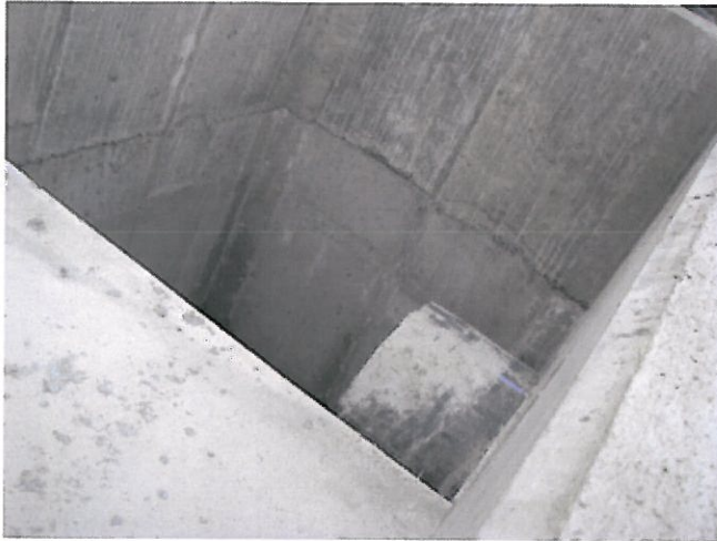
PHOTO 7: BYPASS PARSHALL FLUME OUTLET CHAMBER
