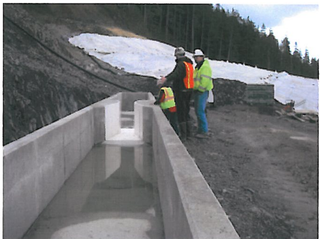
PHOTO 6: PARSHALL FLUME WILL CARRY DIVERTED FLOW
