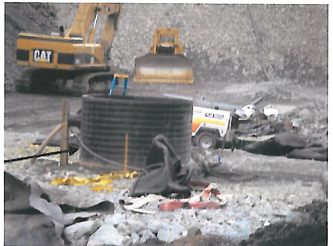
PHOTO 12: SEEP COLLECTION SYSTEM
