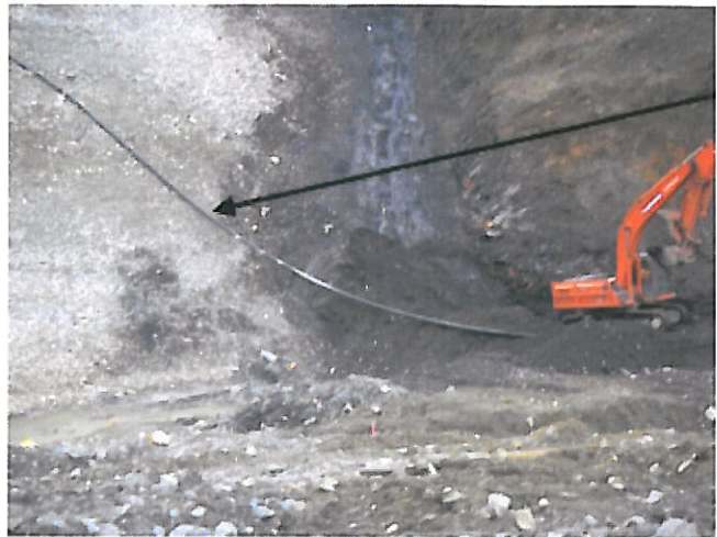
PHOTO 2: BLACK PIPE CONVEYS WATER FROM SEEP COLLECTION SYSTEM TO LOWER SLATE LAKE (TTF).
