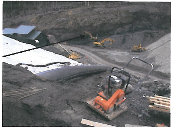
PHOTO 8: HYDRAULIC HAMMER CHIPS (LEFT ARROW) SPILLWAY; LARGE BLACK PIPE IS BYPASS PIPE COMING FROM FROM PARSHALL FLUME
