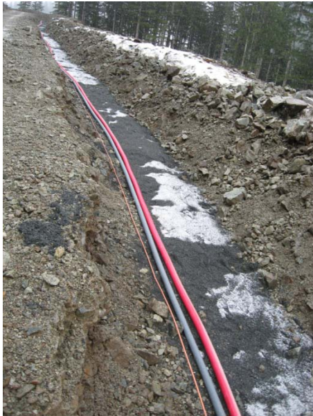
PHOTO 1. FIBER OPTIC AND ELECTRIC CABLES
