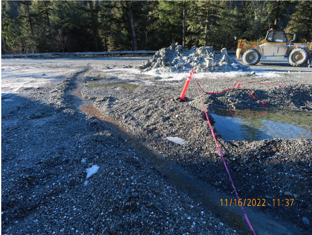
Photo 16. Surface discharge near the abandoned drill casing in Pit 4.
