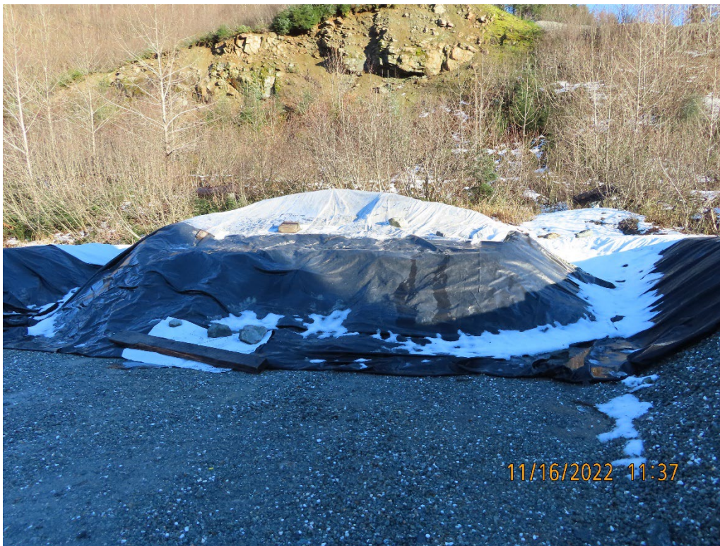
Photo 13. Materials excavated from Wolf ponds that will be shipped offsite for treatment.
