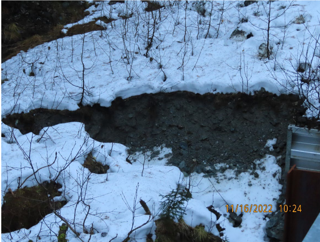
Photo 8. Bank erosion near the Sherman Creek bridge abutment caused by a historic log stringer bridge in Sherman Creek. Coeur Alaska has requested to remove the bridge to prevent further erosion.
