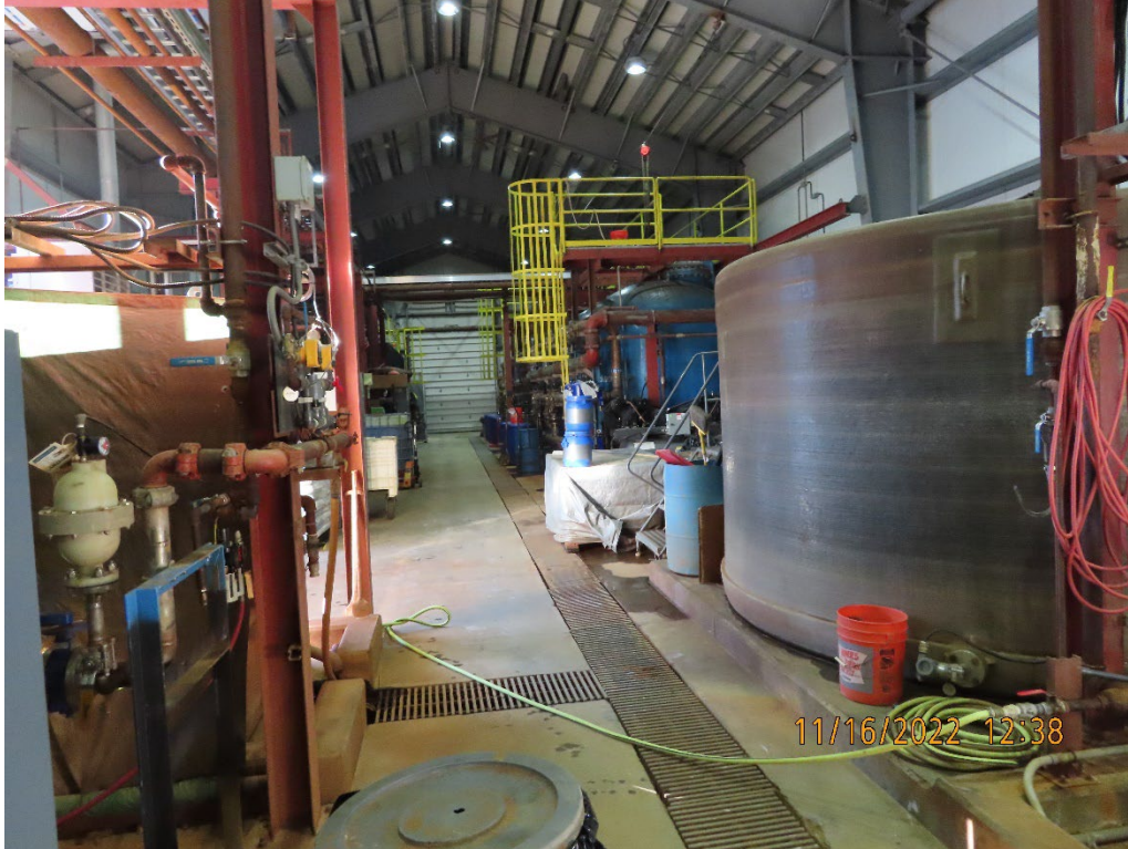
Photo 22. TTF water treatment plant interior.
