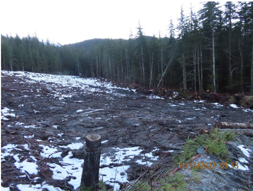
Photo 3. View of the area adjacent to Pond 1 that was cleared and grubbed.
