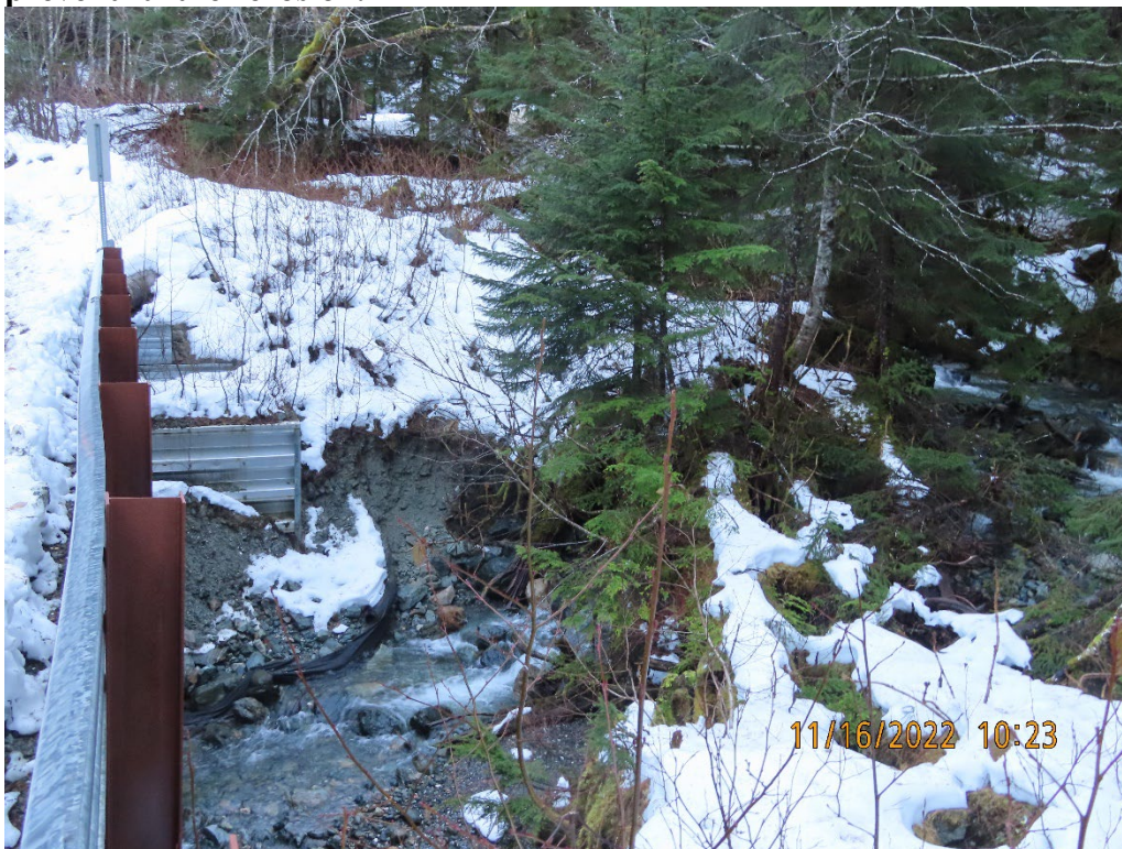
Photo 9. Additional stream bank erosion near the Sherman Creek bridge abutment caused by a historic log stringer bridge in Sherman Creek.
