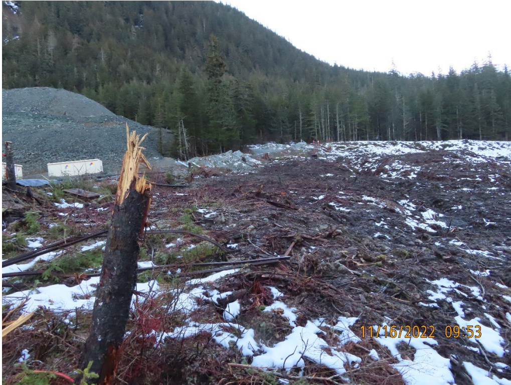
Photo 2. View of the area adjacent to Pond 1 that was cleared and grubbed.
