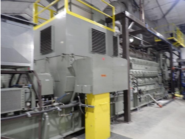
Photo 8. One of four new 4.0-megawatt generators.
