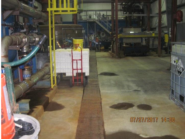
Photo 16. The TTF water treatment plant.
