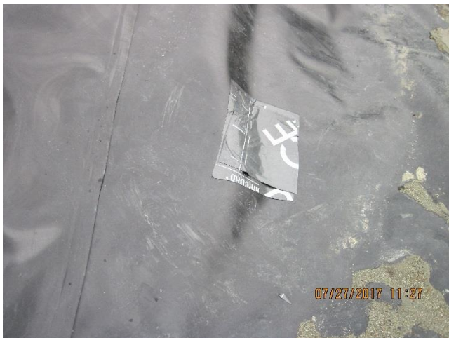
Photo 12. The patches covering the hole where water was pumped out.
