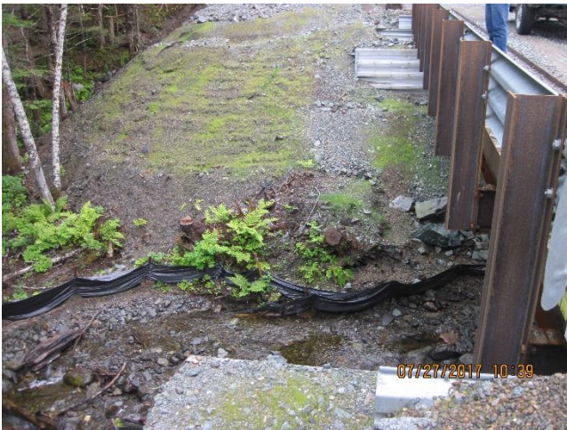
Photo 8. There is sediment buildup along a section of silt fencing at South Fork Sherman Creek Bridge.
