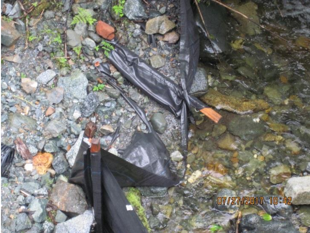
Photo 7. Silt fencing for the South Fork Sherman Creek Bridge is pushed over.
