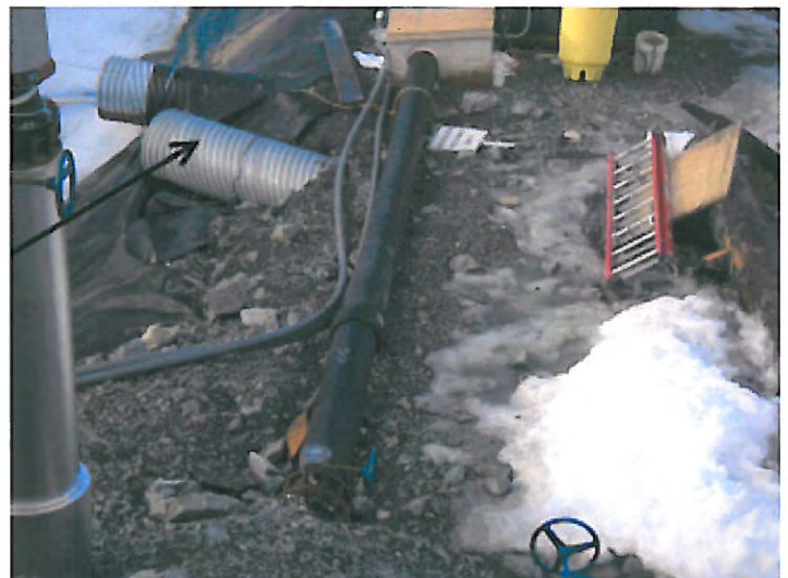
PHOTO 12: ARROW POINTS TO POND 2 OVERFLOW. BLACK PIPE CONVEYS EFFLUENT TO COMPOSITE SAMPLER
