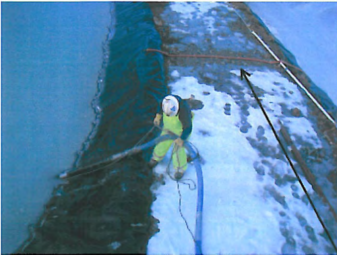
PHOTO 9: PERSONNEL USE EQUIPMENT TO PUMP SEDIMENT FROM POND 1. SEE HOSE HIGHLIGHTED BY ARROW
