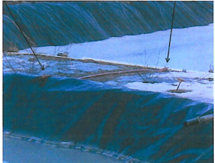
PHOTO 10: HOSE APPEARS TO GO FROM POND 2 TO POND 1
