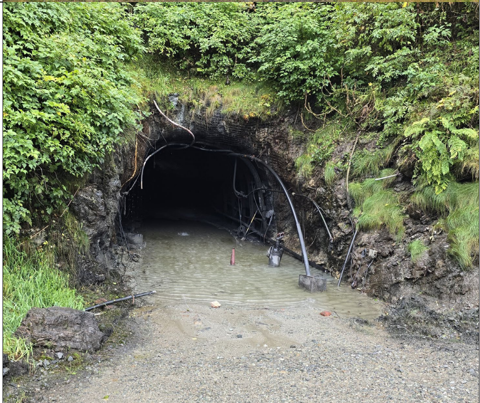
Photo 2: Ponded water observed at the entrance of the 1350 Portal.
