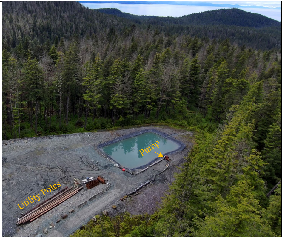
Photo 15: Stormwater pond at Site E with pump used during non-freezing months for runoff management.
