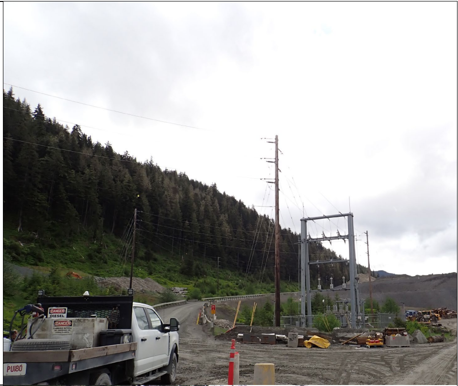
Photo 9: Current power station that will be relocated to a newly cleared pad near A- and B-Roads.
