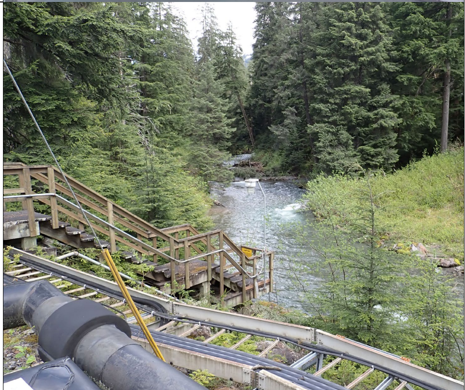
Photo 24: Potable Water Treatment Facility near the 920 Portal. This facility is well maintained. Photo of walkway to one of Greens Creek sampling points.
