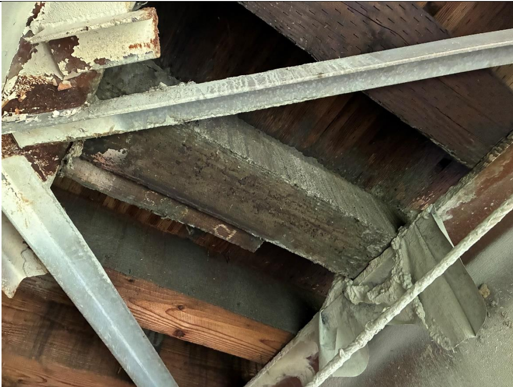
Photo 29: 3.0 Mile B-Road Bridge (Zinc Creek). Sediment potentially leaking through from under the south end decking or residual from before decking was replaced.
