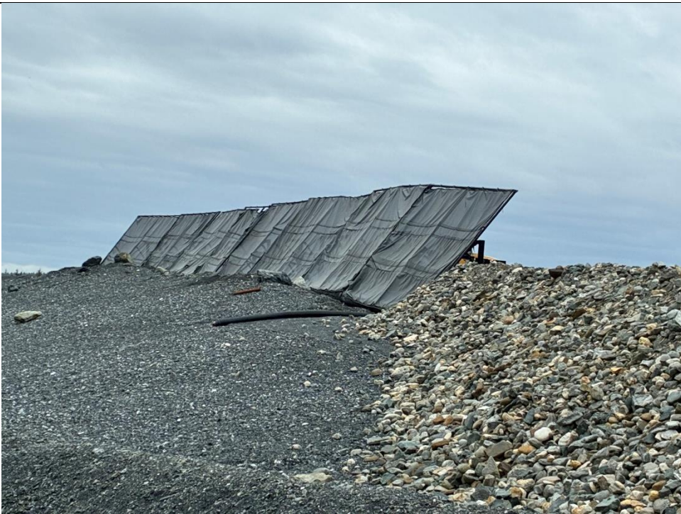
Photo 42: Fugitive Dust Mitigation at the Tailings Disposal Facility.
