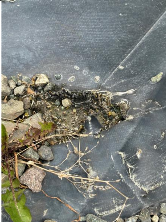
Photo 17: Small tear approximately 6 inches on upper edge of ditch liner from DG-03 to Pond 23.
