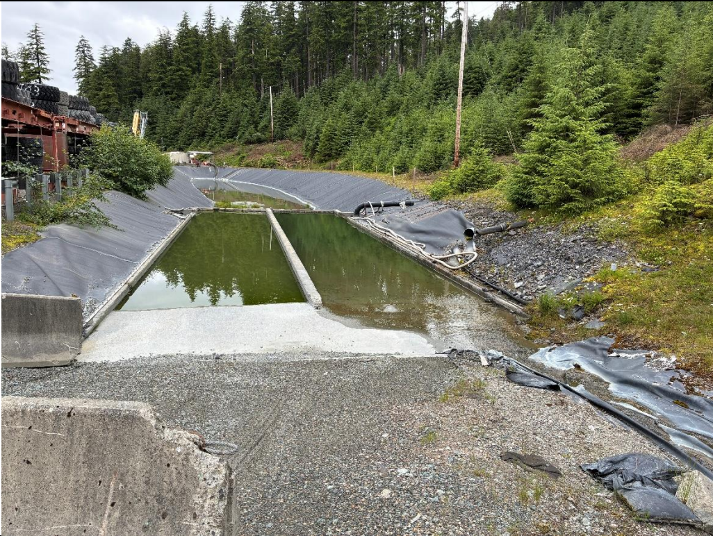
Photo 15: DB-03 and 23 Pond and Pump in background.
