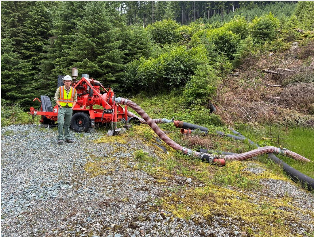
Photo 14: D Pond pump that moves water to Pond 7.
