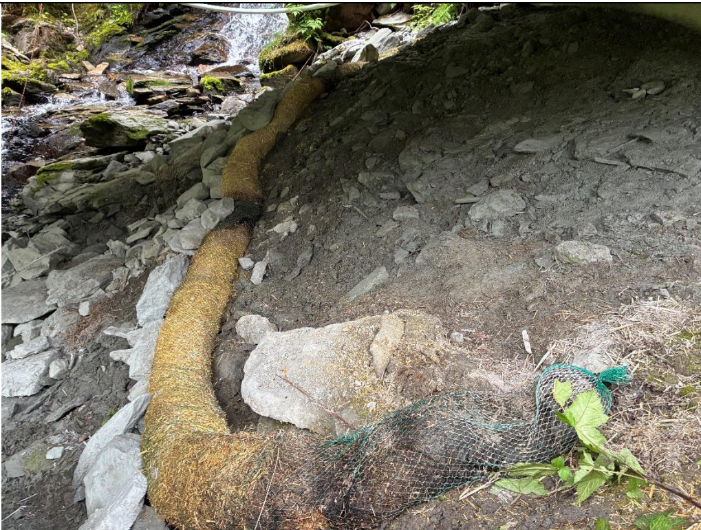
Photo 26: 3.4 Mile B-Road Bridge (Falls Creek) sediment leaking through from under decking.
