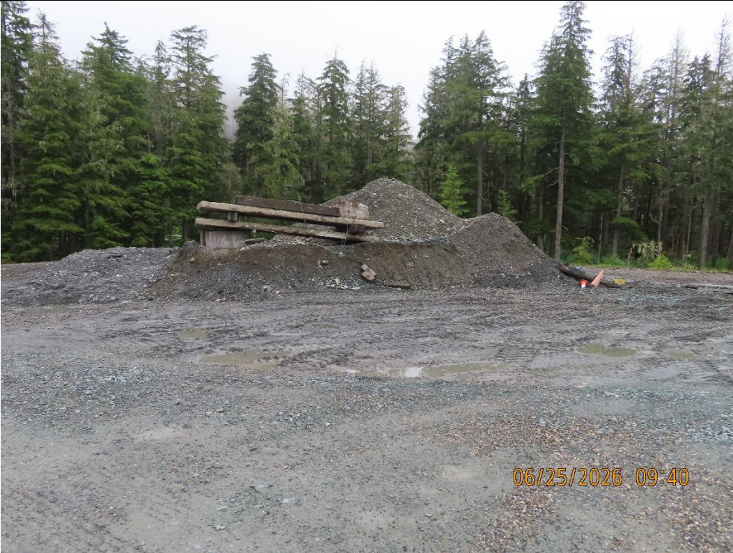
Photo 21: Waste Site E. Much of the material has been moved to the TTF.
