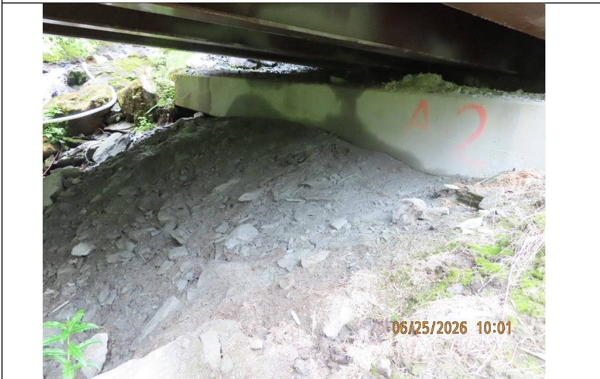
Photo 24: 3.4 Mile B-Road Bridge (Falls Creek) sediment leaking through from under decking.
