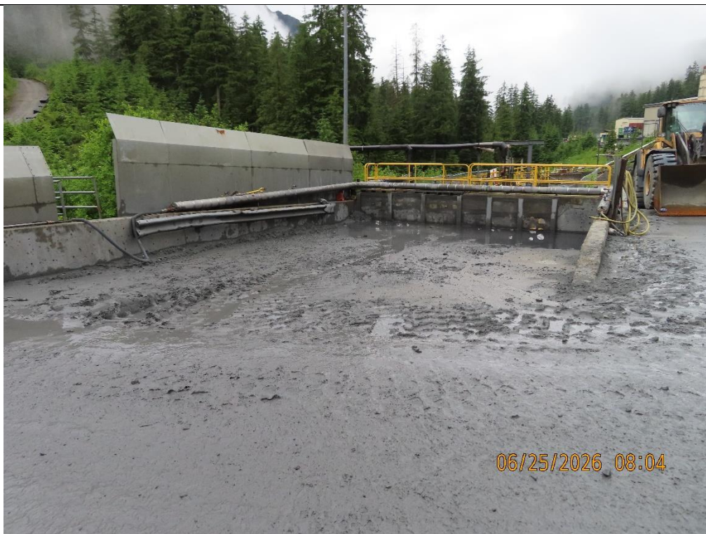
Photo 4: Degrit Basin (DB-01).
