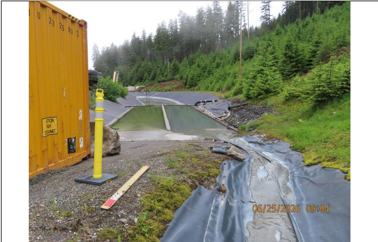
Photo 15: DB-03 and 23 Pond and Pump in background.
