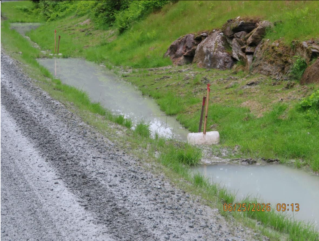
Photo 17: Flocculant log in ditch near 7.4 Mile Bridge.
