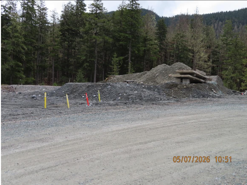
Photo 17: Waste Site E. Much of the material has been moved to the TTF.
