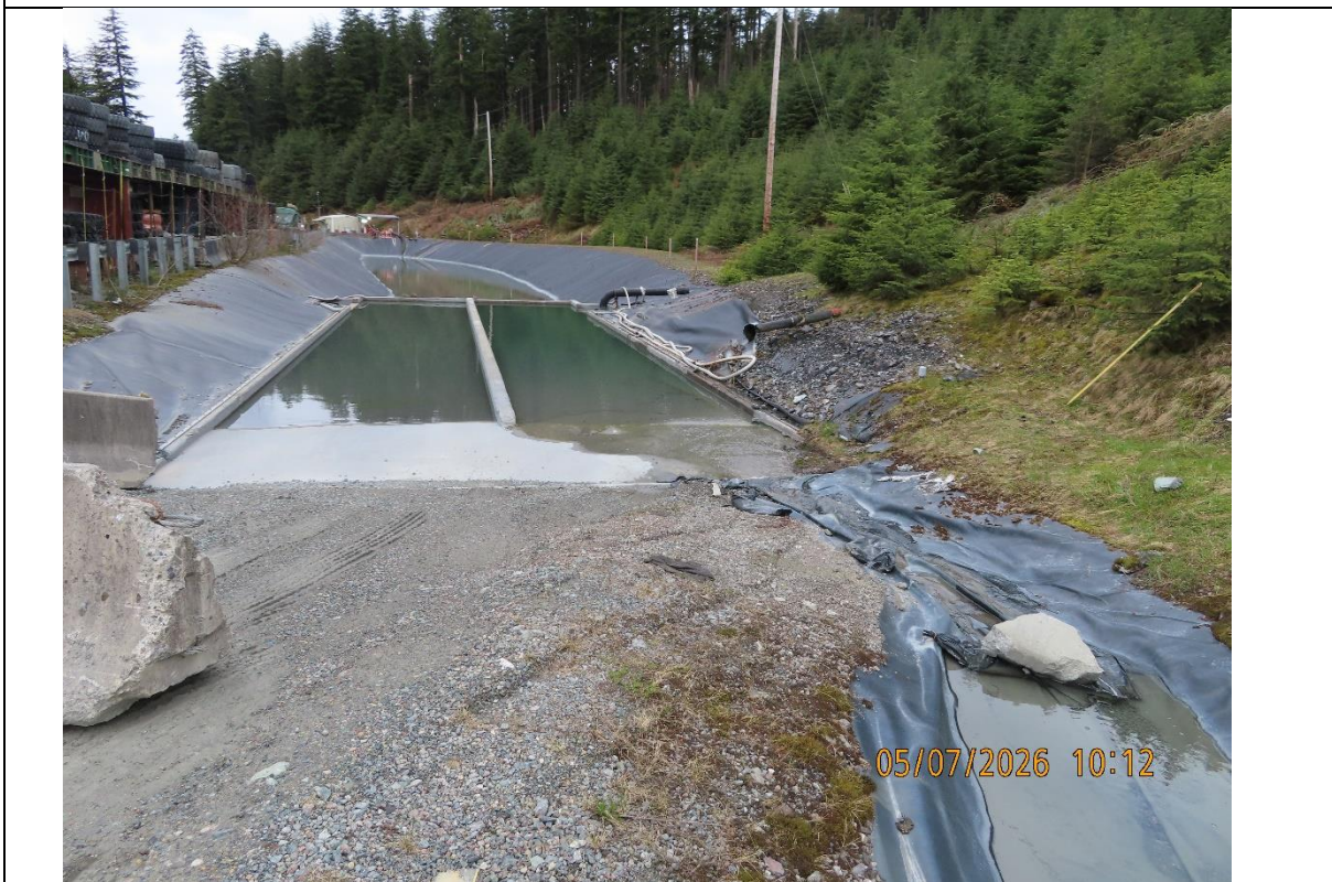
Photo 12: DB-03 and 23 Pond and Pump in background.
