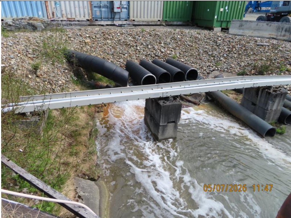
Photo 29: Pond 7 receiving tailings and water from tailings pile and Pond 9.
