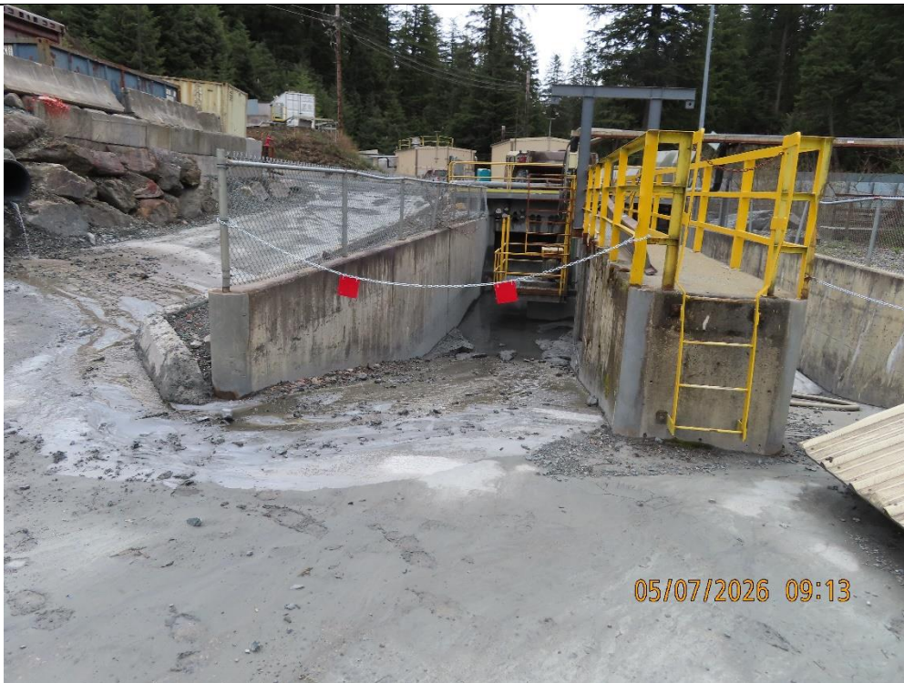
Photo 4: Degrit Basin (DB-01) back side.
