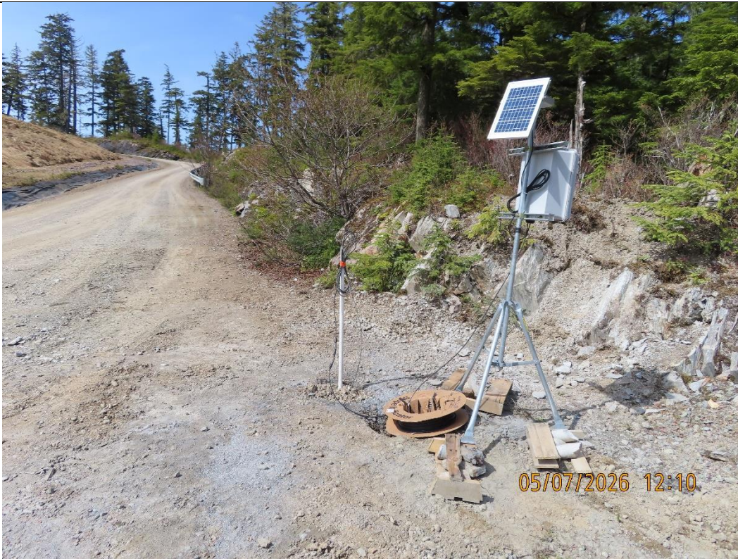
Photo 35: Vibrating wire piezometer (VWP) VWP PZ-T_26_01A at the North Expansion Project area.
