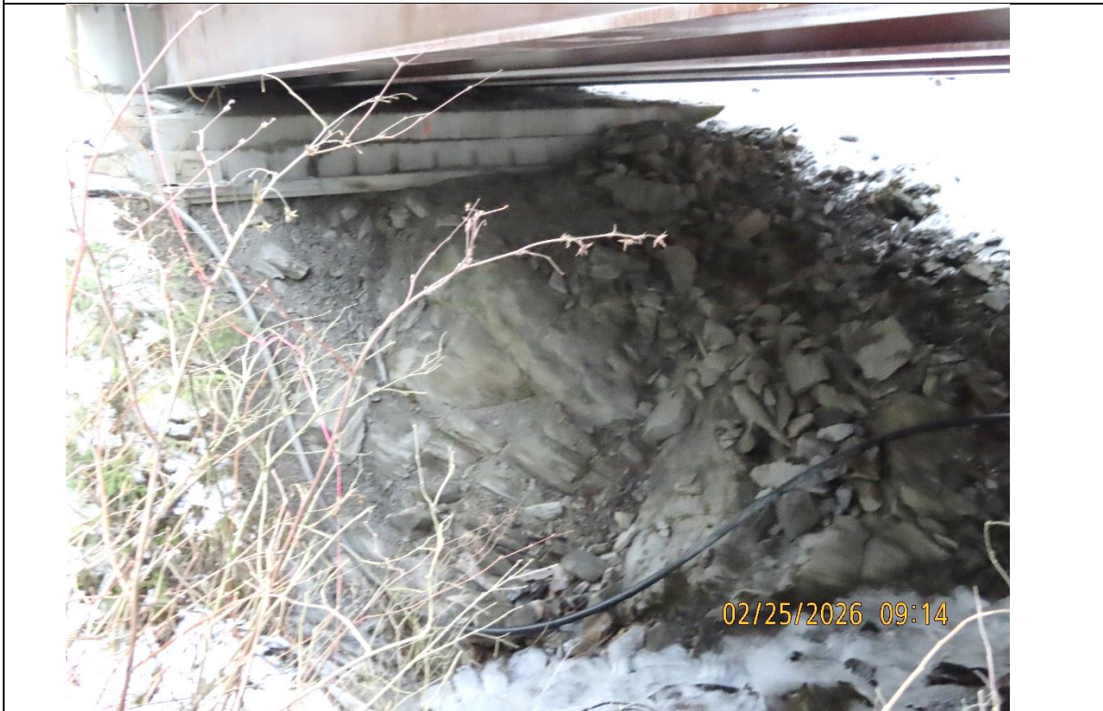
Photo 20: 3.4 Mile B-Road Bridge (Falls Creek) sediment leaking through from under decking.
