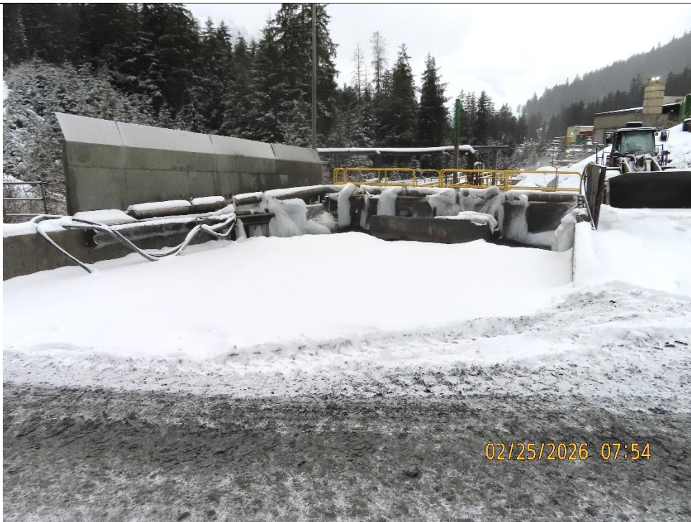
Photo 4: Degrit Basin (DB-01).
