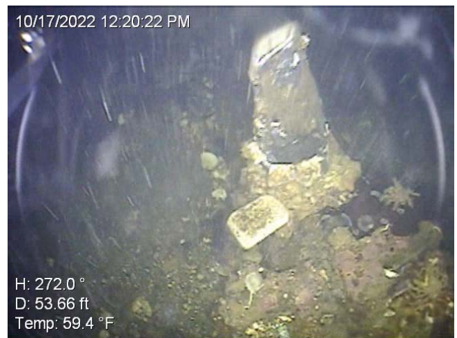
Typical Diffuser Condition
