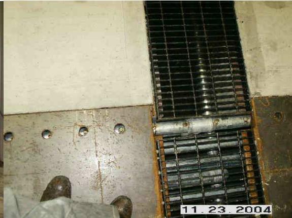
Vertical jets to wash tires & underside of trucks
