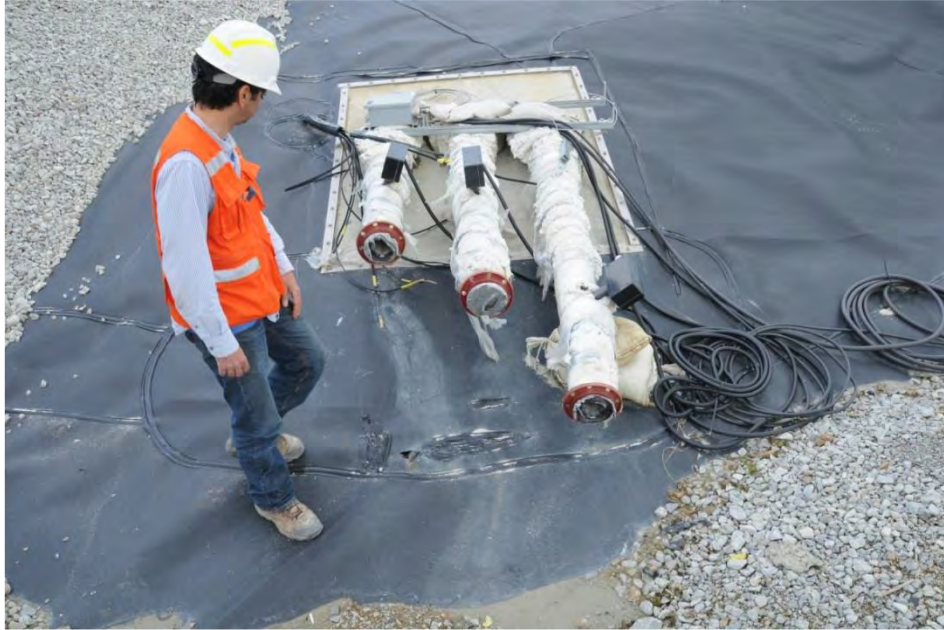
Figure 3-10 – Close-up View of the PCMS Outlets
