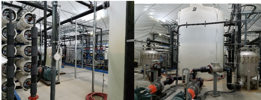
Reverse Osmosis Water Treatment Plant (RO2)
