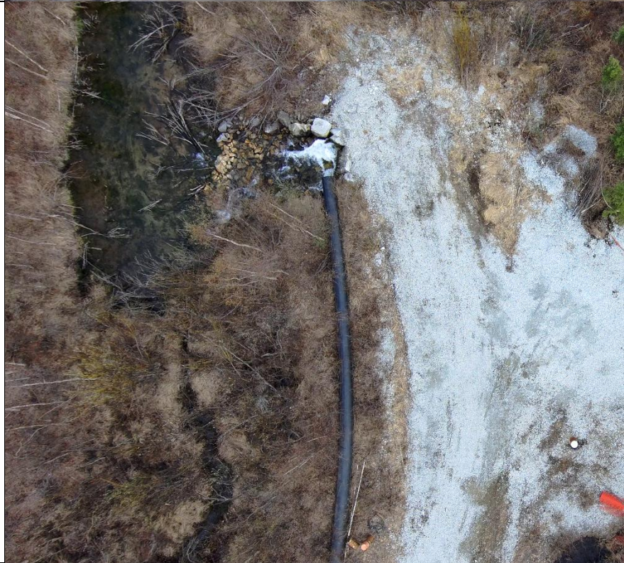
Photo 26: Treated water discharging from RO2 into the wetlands complex and Fish Creek.
