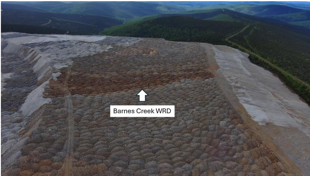
Photo 26: Northeast corner of Barnes Creek Waste Rock Dump. The view is to the south-southwest. Recontouring of the BCWRD was observed.
