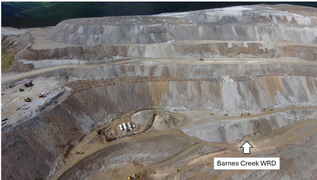
Photo 27: Northeast corner of Barnes Creek Waste Rock Dump. The view is to the west.
