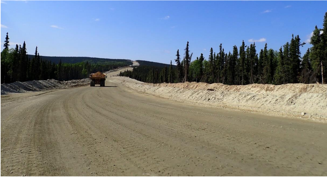
Photo 2: Gil haul road condition and berms.
