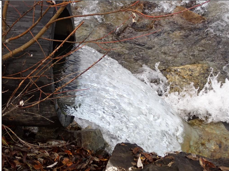
Photo 20: Outfall 002. At the time of inspection, the Outfall was in good condition and the water looked clear and clean.
