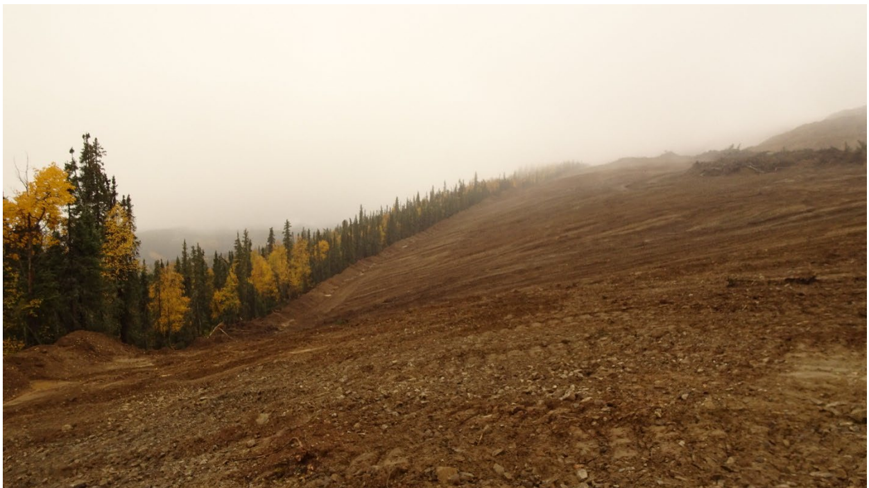
Edge of striping of vegetation for the Victoria Creek waste rock dump.
