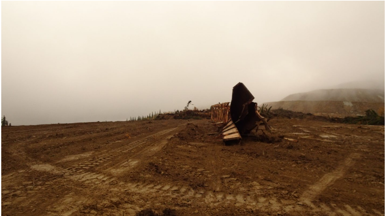
Old sluice box exposed while stripping overburden for Victoria Creek waste rock dump
