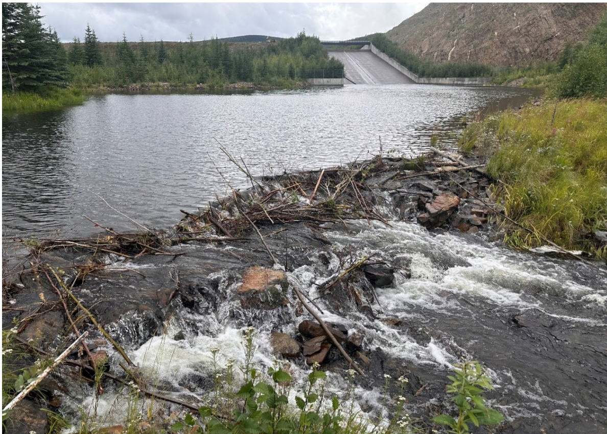
Figure 5. Stilling Basin outlet beaver dam, August 1, 2024.
