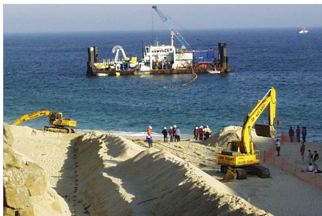
Fig. 4. Installation works of the 2000 FLAG Atlantic 1 in the intertidal area, Brittany, France (courtesy: www.ldravocean.fr).
