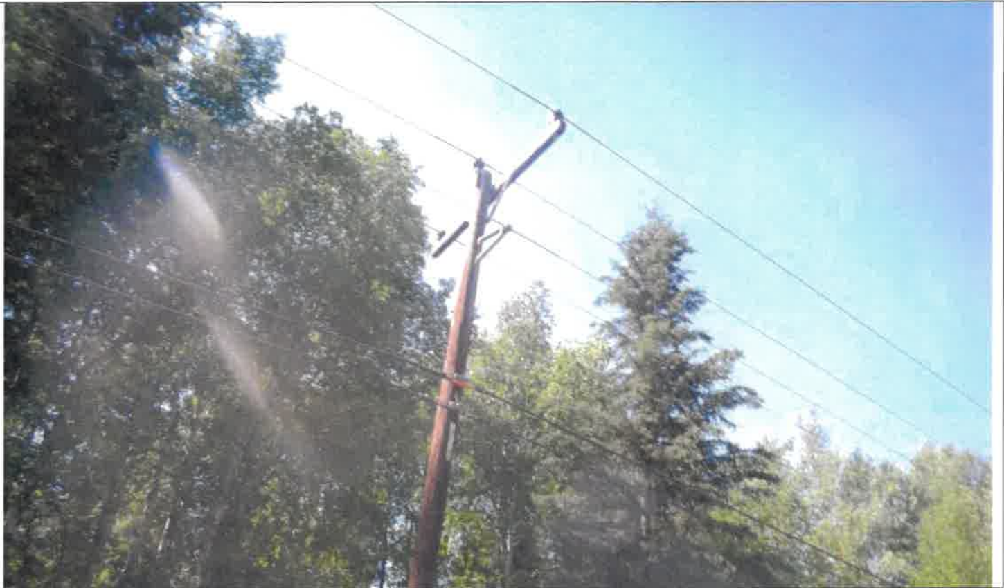
Overhead powerline on the eastern lot line of Tract A. File photo.
